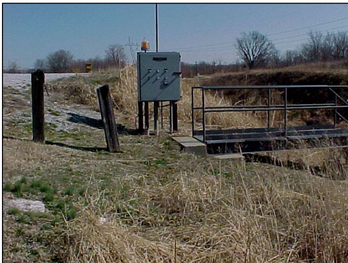
Photo 33 Outfall 010 Lift Station
