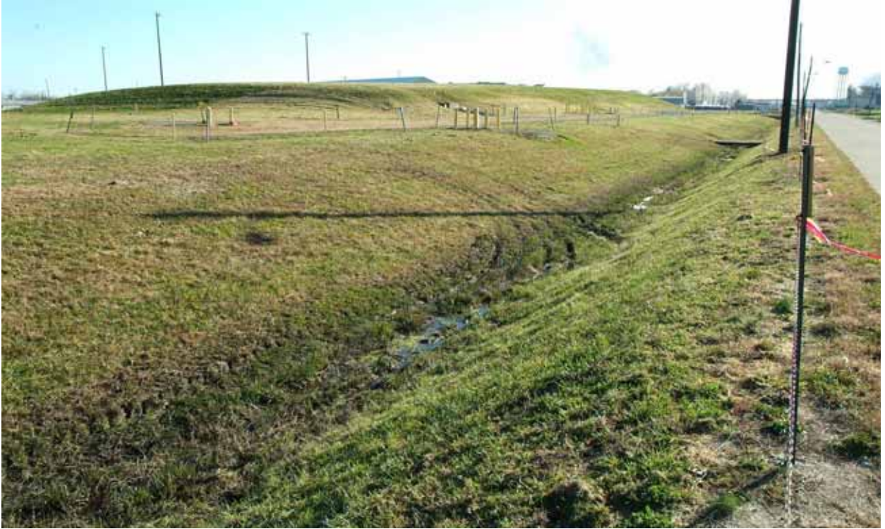
Figure E.15. Outfall 015 EU03 11-12-09 (Before)
