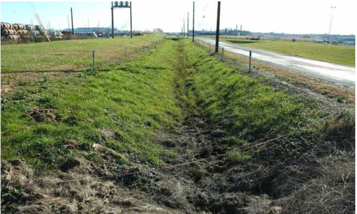
Figure E.14. Outfall 015, EU02 11-12-09 (Before)
