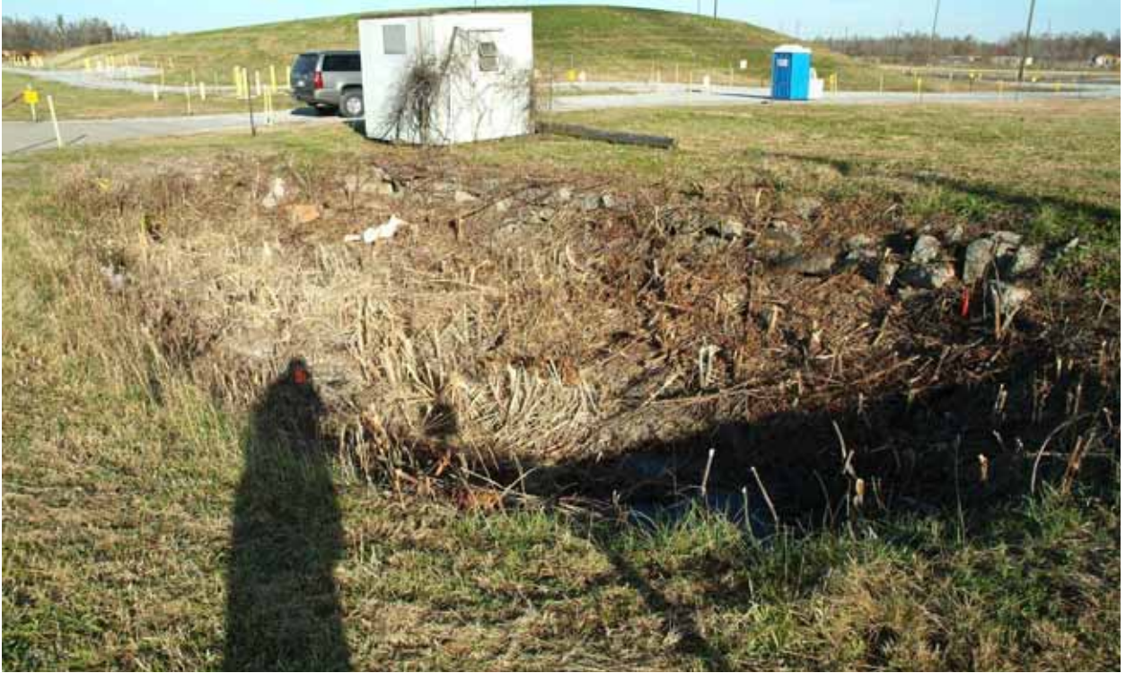
Figure E.17. Outfall 015 EU04 11-12-09 (Before)
