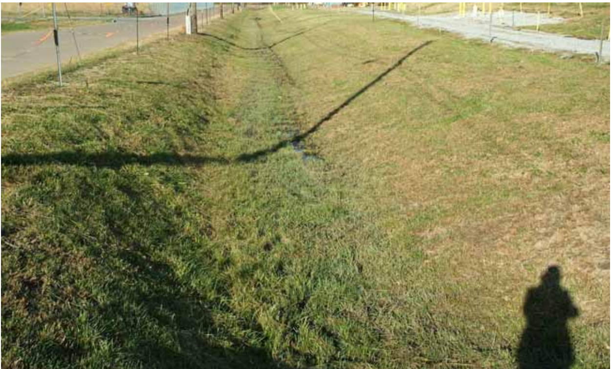
Figure E.16. Outfall 015 EU03 11-12-09 (Before)
