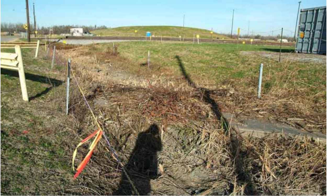
Figure E.19. Outfall 015 EU04 11-12-09 (Before)
