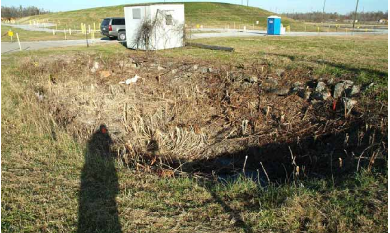
Outfall 015 EU04 11-12-09 (Before)
