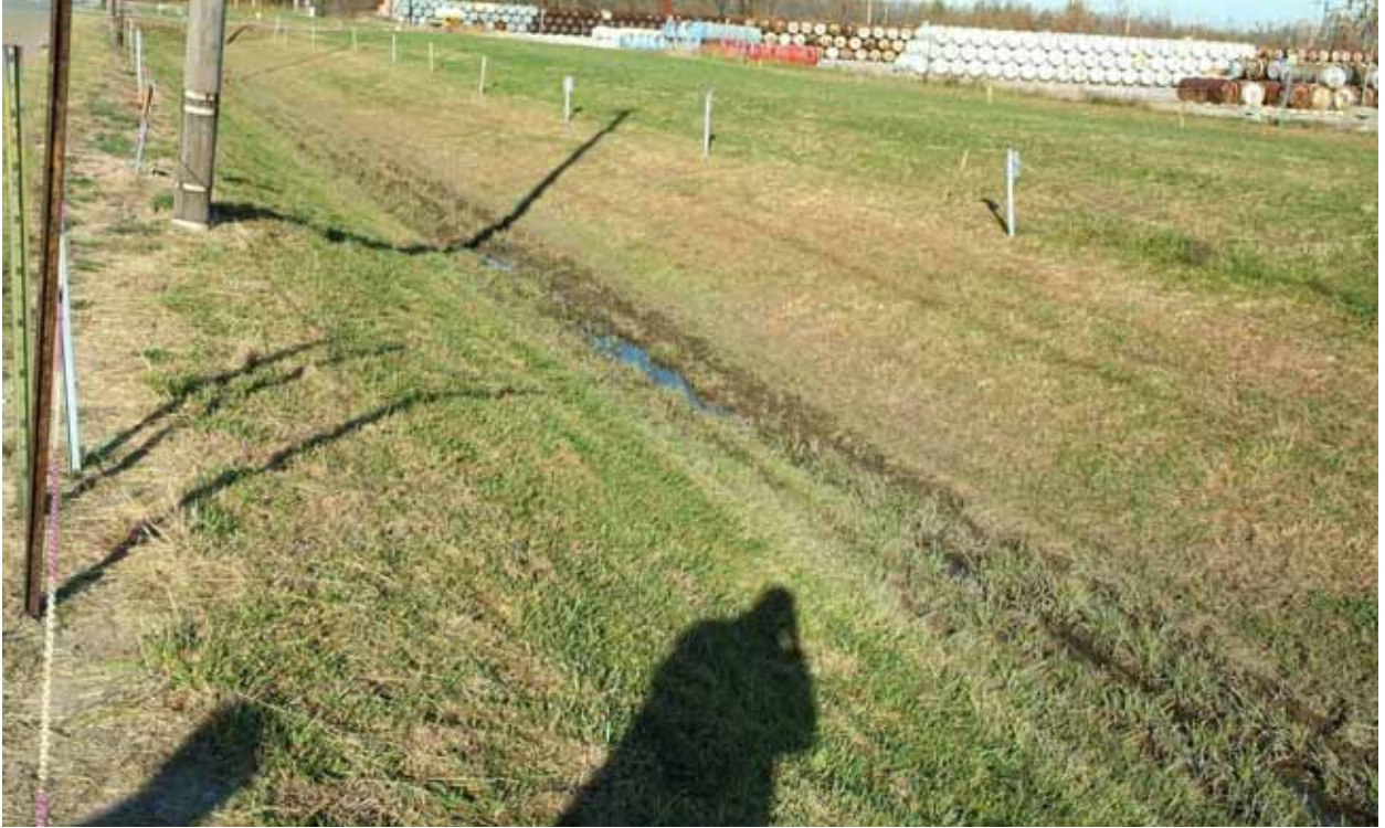
Outfall 015, EU02 11-12-09 (Before)
