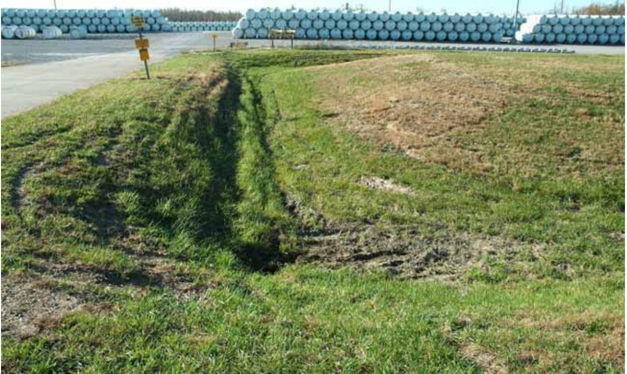
Outfall 015 EU08 11-12-09 (Before)
