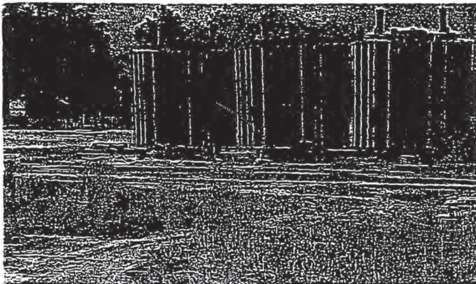
Large electrical transformers at the site—a former transformer rehabilitation and storage facility
