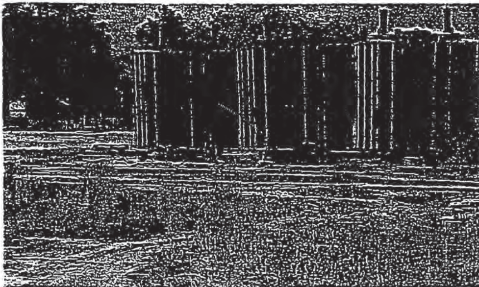
Large electrical transformers at the site—a former transformer rehabilitation and storage facility
