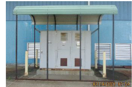
300 kVa, 14 kv/480V Dry-type Transformer
