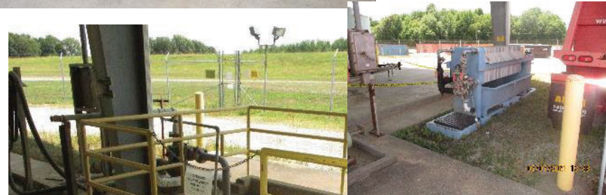
Poly wastewater storage tanks and a geobag and filter press
