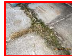
Cracks with grass
