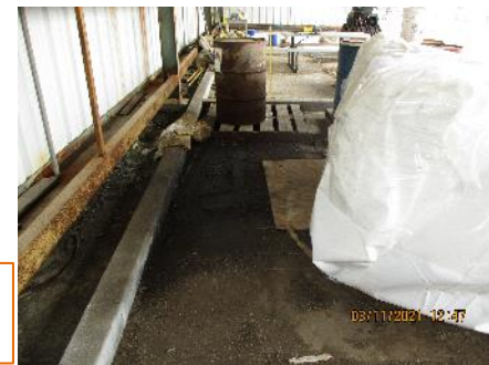
Bay 5 – North to South Floor Staining
