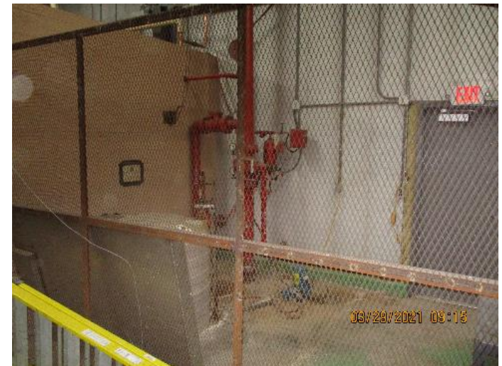
Photo (3/2021) of Sodium Thiosulfate Chemical Feed Station.
