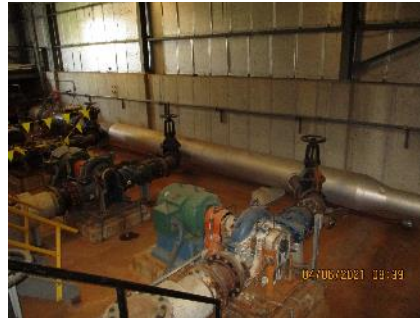
Pump Discharge Header
