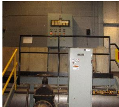
Pump Control Panel
