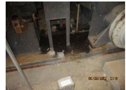
C-631-4 - Oil Staining
