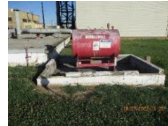
C-631-3 – Diesel Fuel Tank
