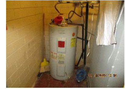
C-631-1 - South Wing Water Heater
