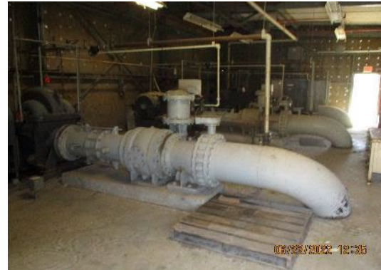
C-631-4 - Pump Discharge Lines
