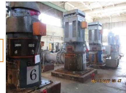
C-631-1 - Center Structure Pumps
