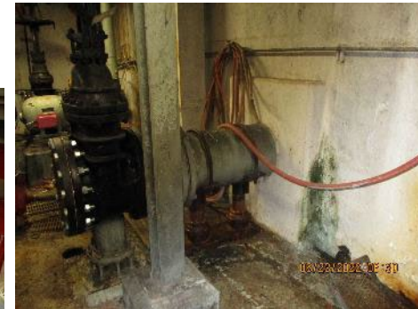
C-631-3 - Pump House (Firewater) Interior View – Pump #3 Suction
