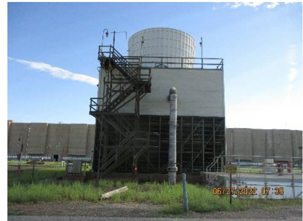
C-631-6 Blending Cooling Tower - South Side
