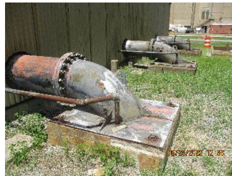
C-631-4 - Pump Suction Lines Exterior View
