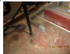
Gray pipe from chemical area feeding into to wet well
