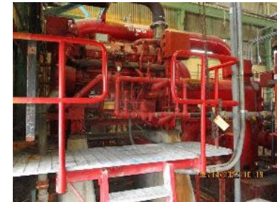
C-631-1 - Center Wing High Pressure Fire Water System
