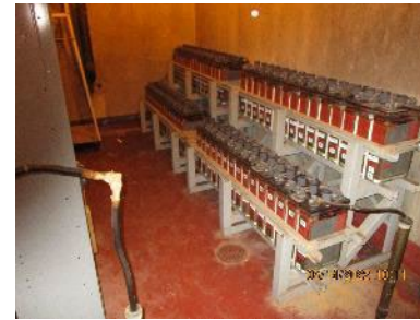
C-631-1 – South Wing Lead Calcium Batteries
