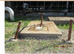
B-Loop Return to Blending Tower Vault
