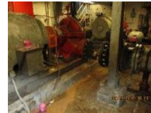
C-631-3 - Oil Staining
