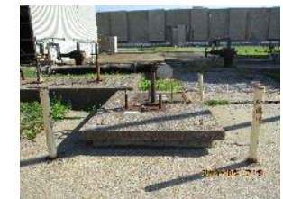
C-631-2 - Surrounding Area Vaults and East Basin Pad
