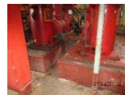
C-631-1 - Center Structure HPFWS Pump Oil Stain
