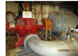
C-631-3 – No. 3 HPFWS Pump and Motor
