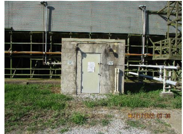
C-631-2 Sprinkler System - External View
