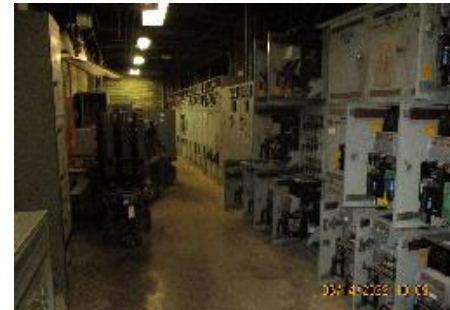
C-631-1 - South Wing Interior Switchgear Room
