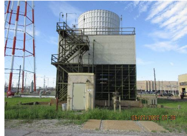
C-631-6 Blending Cooling Tower – North Side
