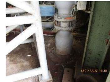
C-631-1 - Center Structure Pump Relief Surge Entry to Wet Well
