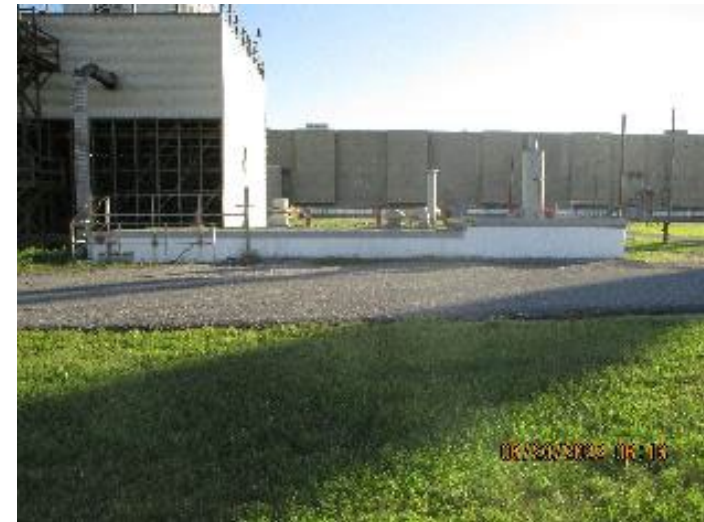
C-631-3 - Pump House (Firewater) South Side
