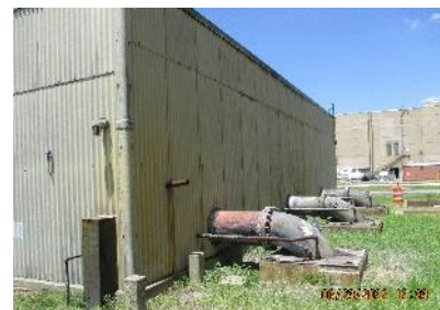
C-631-4 – Blending Pump House East Side
