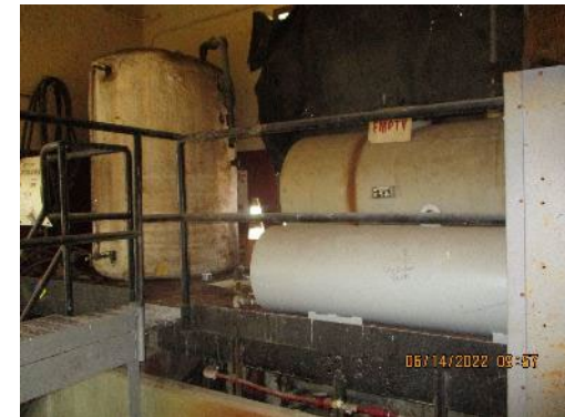
C-631-1 North Wing Sulfuric Acid Pig and Tanks
