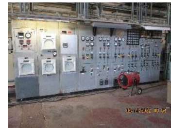
C-631-1 - Center Structure Control Panel
