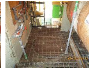
C-631-1 - North Wing Platform –Historical Location of 185-gal chromate-soda ash solution Tank
