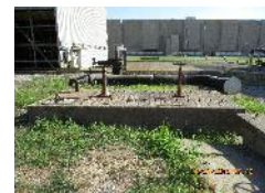
A-Loop Return and Bypass Vault (Valve Vault B)
