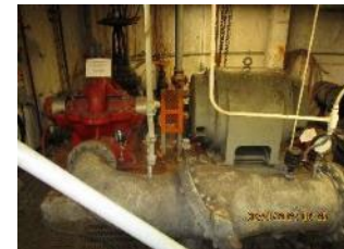
C-631-3 – No. 2 HPFWS Pump and Motor
