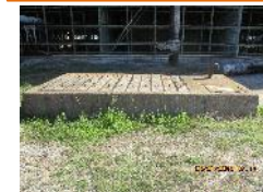
B-Loop Return Vault (Valve Vault A)
