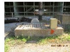
Make-up Water Venturi Vault (Valve Vault F)
