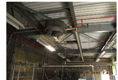
C-631-4 – Ceiling Ventilation and Steam Heater
