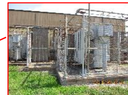
External Electrical Transformers
