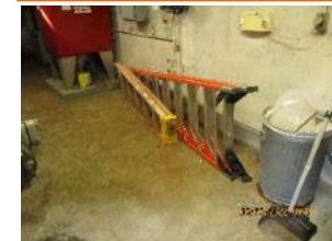
C-631-3 – Loose Equipment
