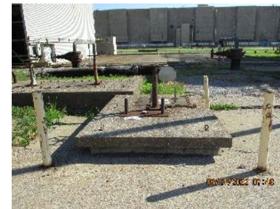
A-Loop Return Vault to C-631-6 Blending Tower
