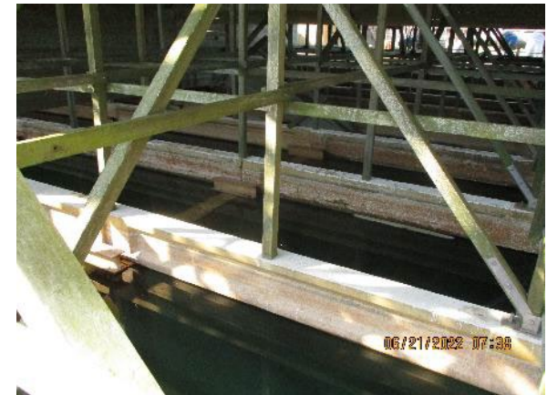
C-631-2 Cooling Tower – Interior View
