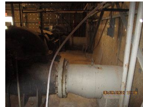
C-631-4 - Pump Suction Line Interior View
