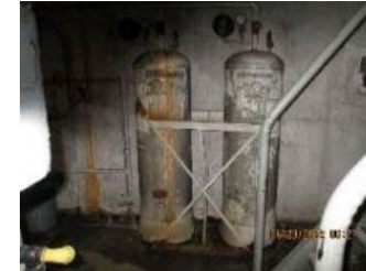
C-631-3 – Diesel Air Tanks
