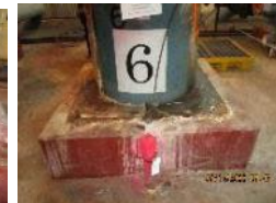
C-631-1 - Center Structure Pump Oil Stain
