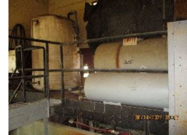
C-631-1 - North Wing Sulfuric Acid Pig and Tank
