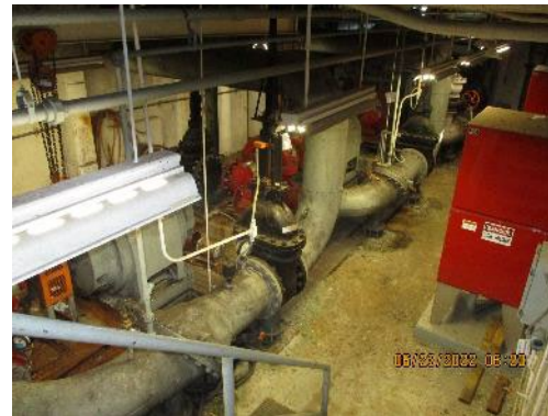
C-631-3 - Pump House (Firewater) Interior View Looking East
