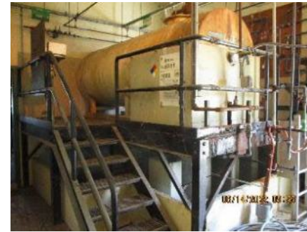
C-631-1 - North Wing Calgon Room (Corrosion Inhibitor Feed Area)
