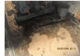
C-631-3 - Water Staining
