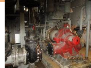
C-631-3 – No. 4 HPFWS Pump and Diesel Motor
