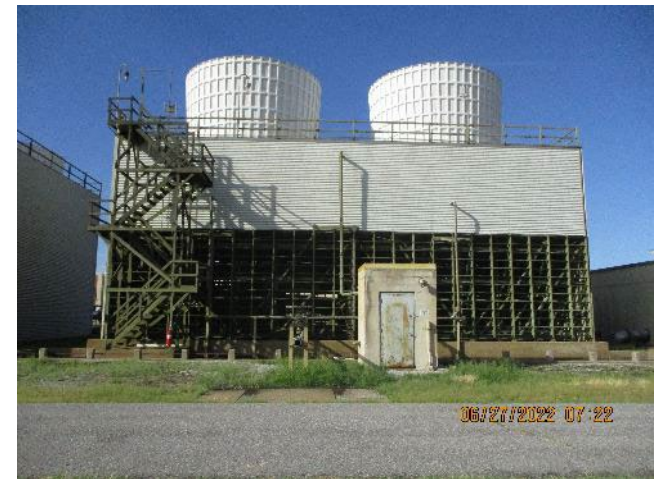
C-631-5 Blending Cooling Tower – North Side
