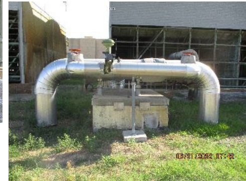
C-631-2 Plant Water Station
