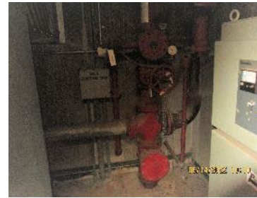
C-631-1 - South Wing Transformer Sprinkler System
