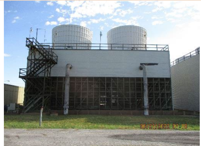
C-631-5 Blending Cooling Tower – South Side
