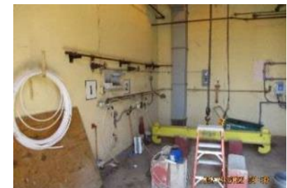
C-631-1 - North Wing Chlorine Feed Header
