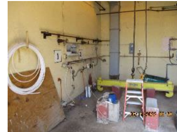
C-631-1 - North Wing Chlorine Area
