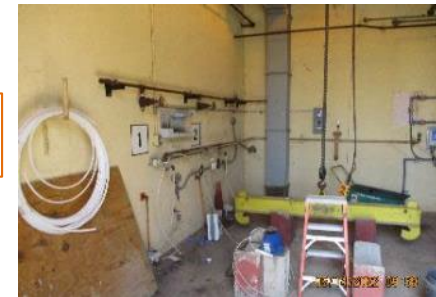
C-631-1 - North Wing Chlorine Feed Header
