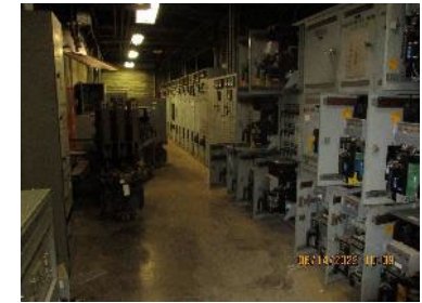
C-631-1 – South Wing Switchgear Room – Looking East
