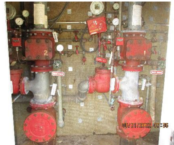
C-631-2 Sprinkler System - Internal View
