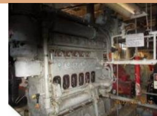
C-631-3 – No. 4 HPFWS Pump Diesel Engine
