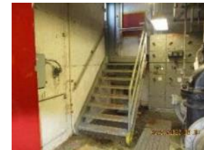
C-631-3 – South Door and Electrical Panel
