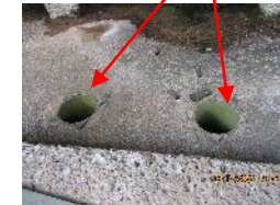
9-inch Diameter Holes to Basin (Allows cooled RCW water to fall into the basin below)
