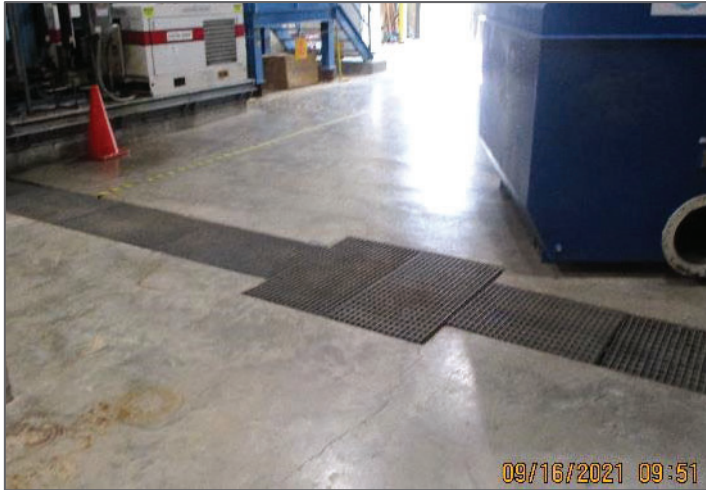
Floor Drain with Sump
