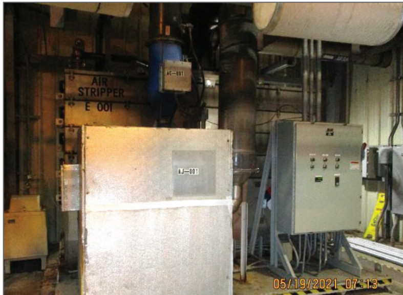
Air Stripper and Controls
