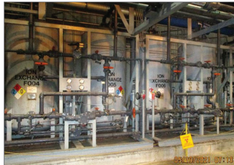
Formerly used Ion Exchange Tanks/Columns (Posted as a Radioactive Material Area)
