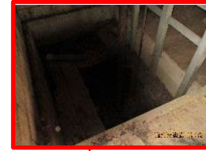
Pump Pad Area
