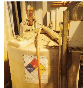
Sodium Thiosulfate unit
