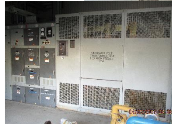
Substation Transformer South End
