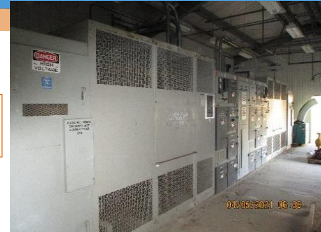
Substation Transformer North End
