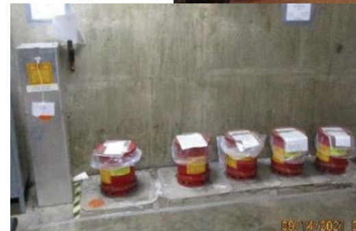
Sump pump/pit in the basement floor of the mechanical room (right)
