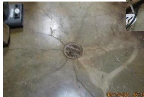
Floor drain (left)
