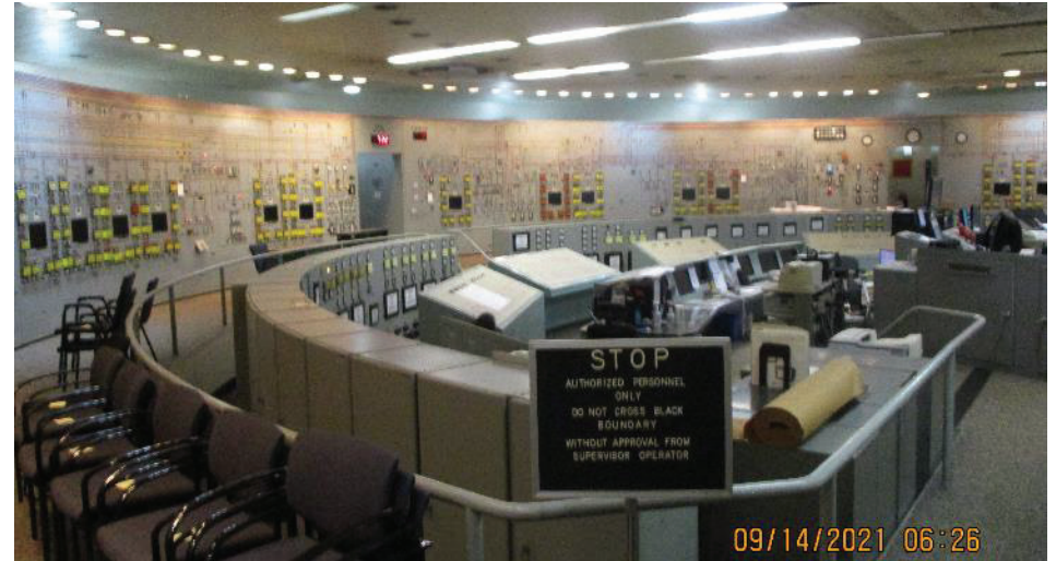
Central Control Room on Main Ground Level Floor
