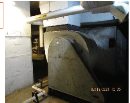
Air Moving Fan in Basement
