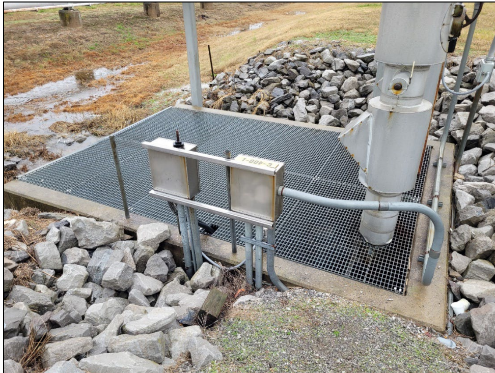
Figure 11.2. C-400-L Lift Station
