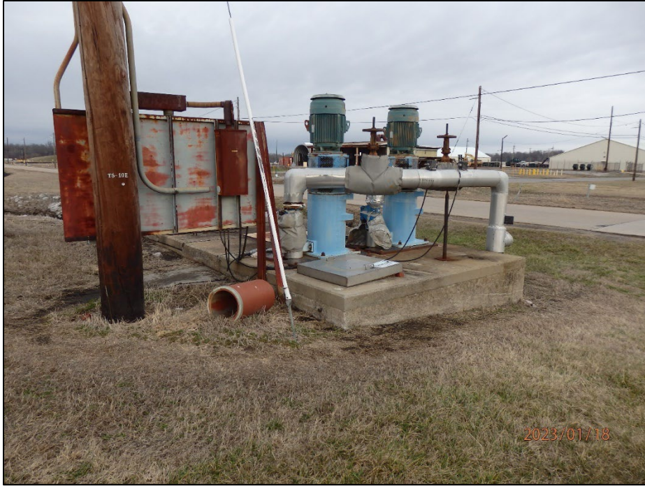
Figure 11.3. C-616-L Lift Station and C-400-L Piping
