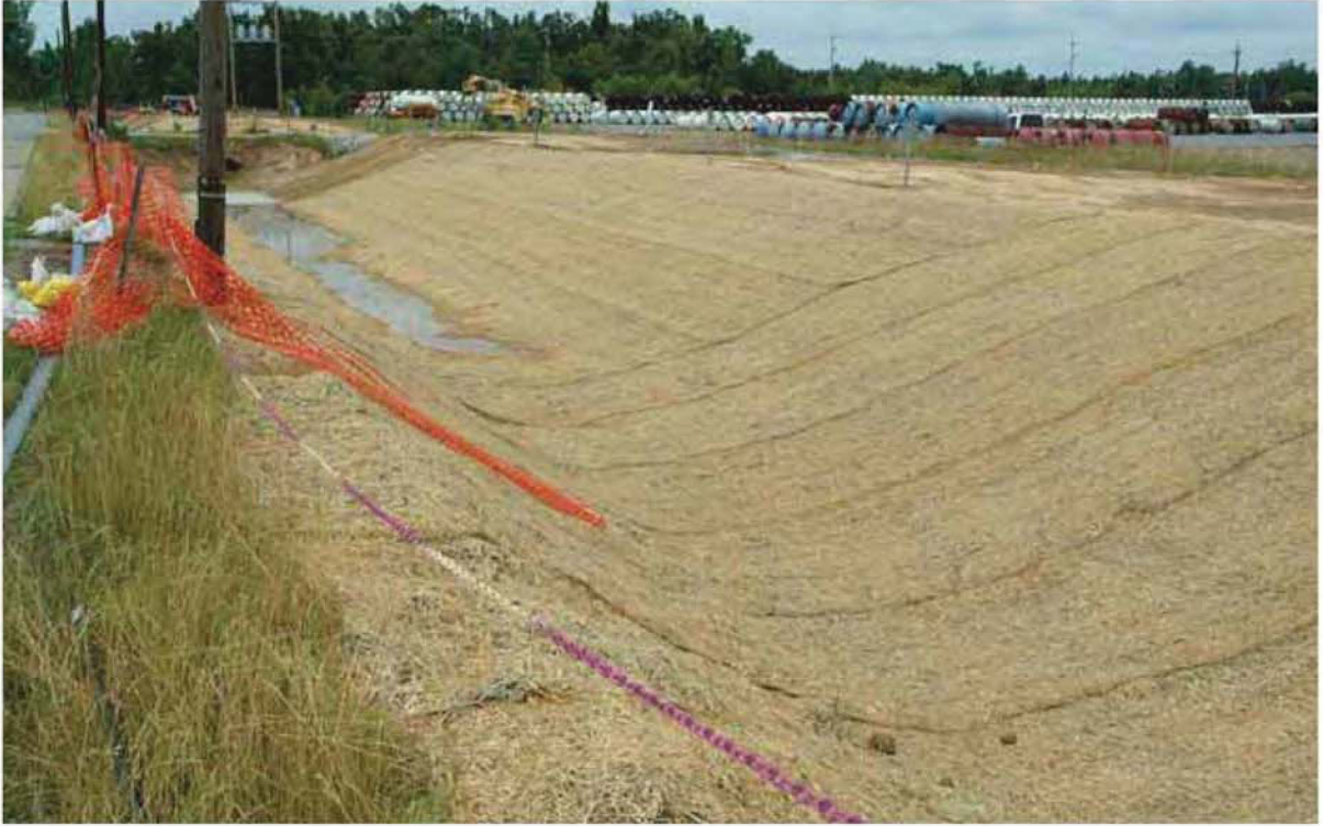
Figure 16.19. Outfall 015, EU 02 07-12-10 (After)
