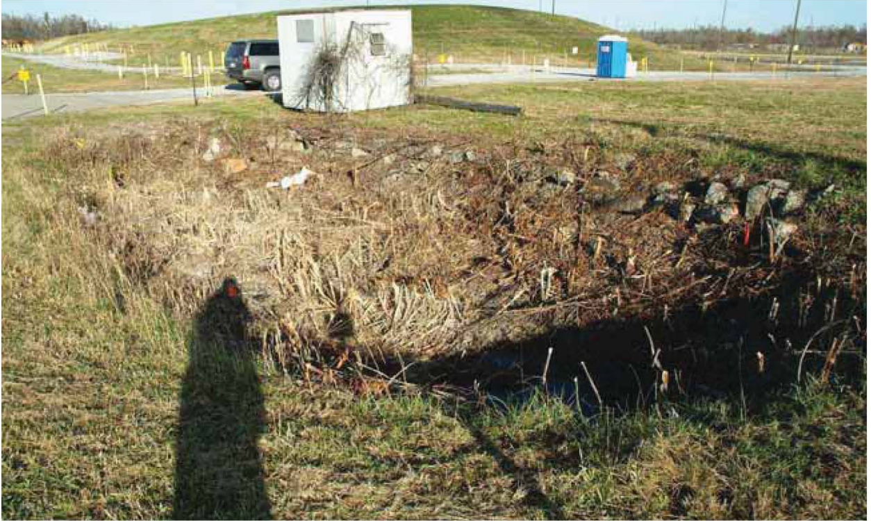
Figure 16.14. Outfall 015 EU04 11-12-09 (Before)
