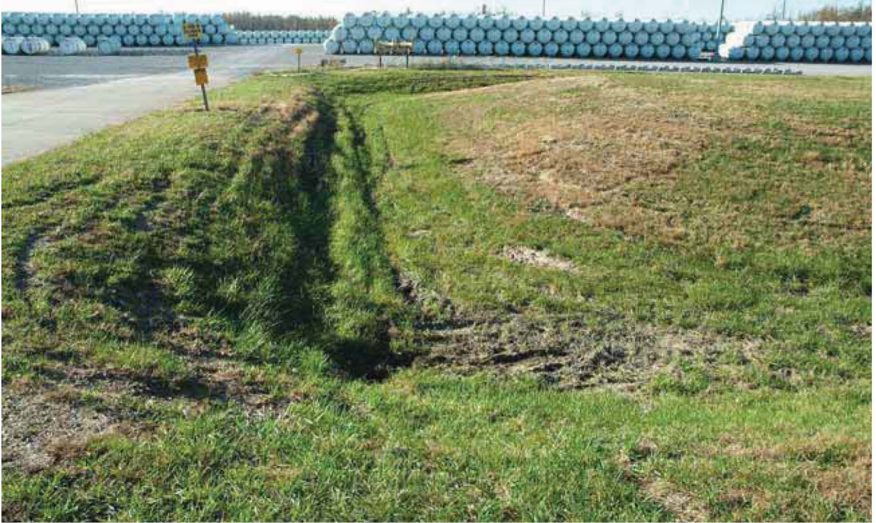
Figure 16.18. Outfall 015 EU08 11-12-09 (Before)
