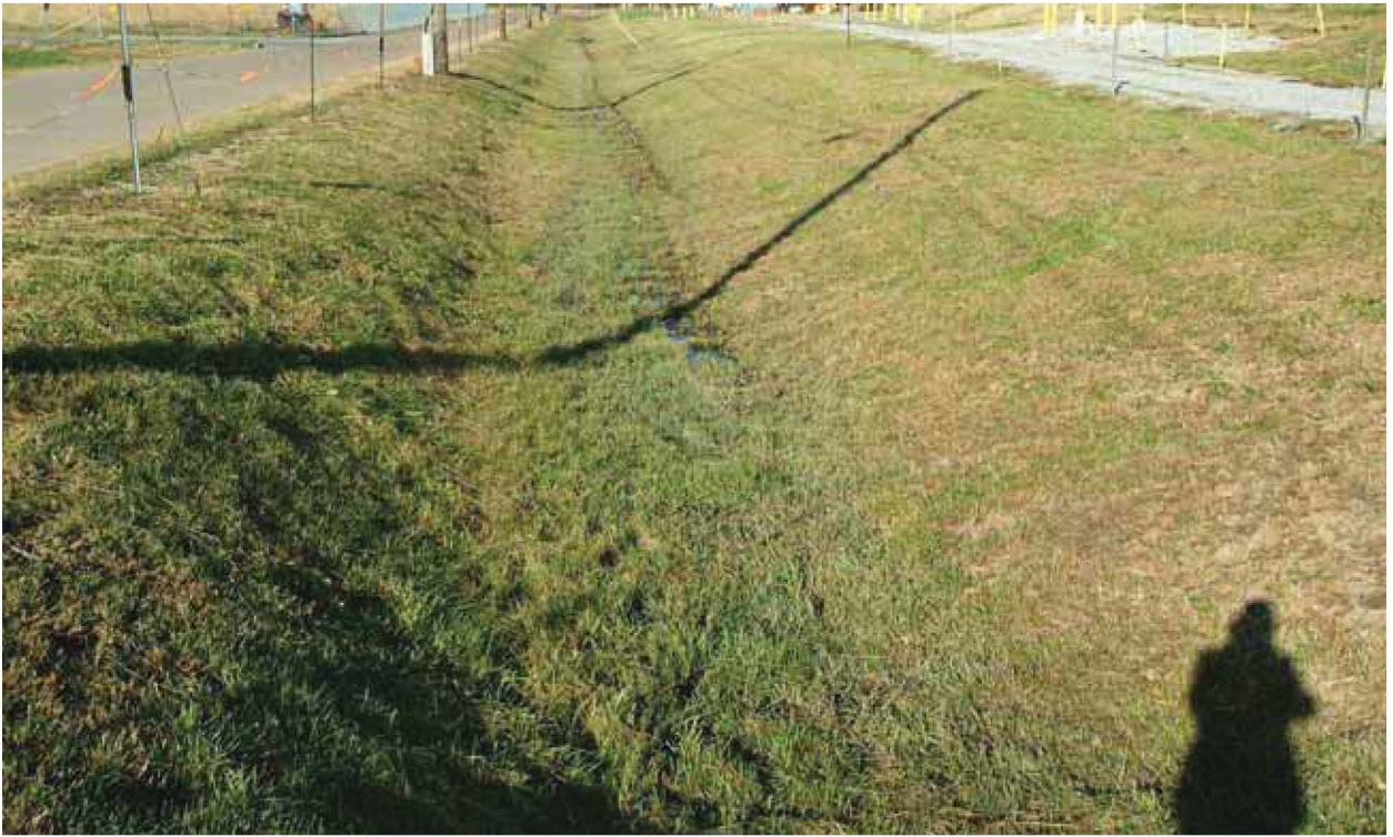
Figure 16.13. Outfall 015 EU03 11-12-09 (Before)
