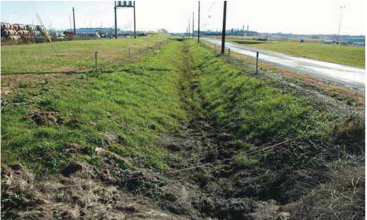
Figure 16.11. Outfall 015, EU02 11-12-09 (Before)
