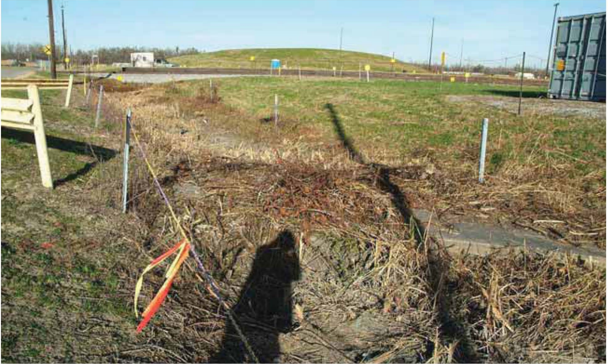
Figure 16.16. Outfall 015 EU04 11-12-09 (Before)
