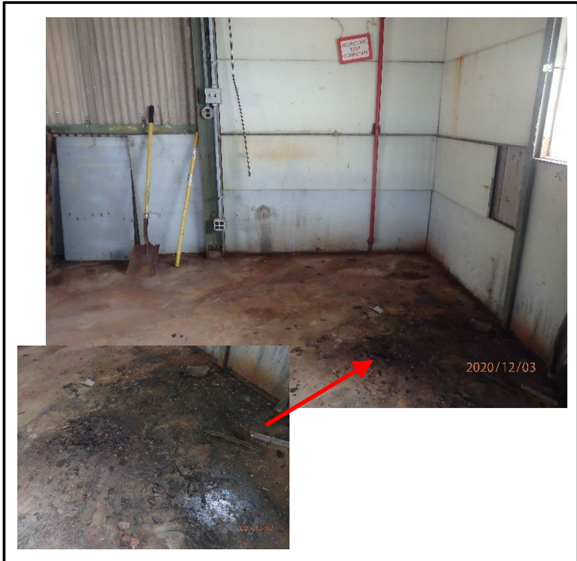
Figure 8. Evidence of Past Spill Staining in C-721
