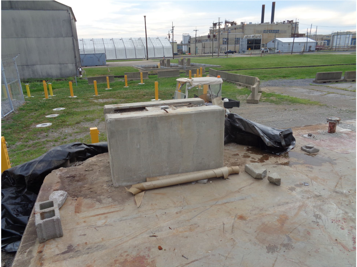
Figure 6. Concrete Structure Surrounding the Steel Cobalt Well on Remaining Slab Facing North
