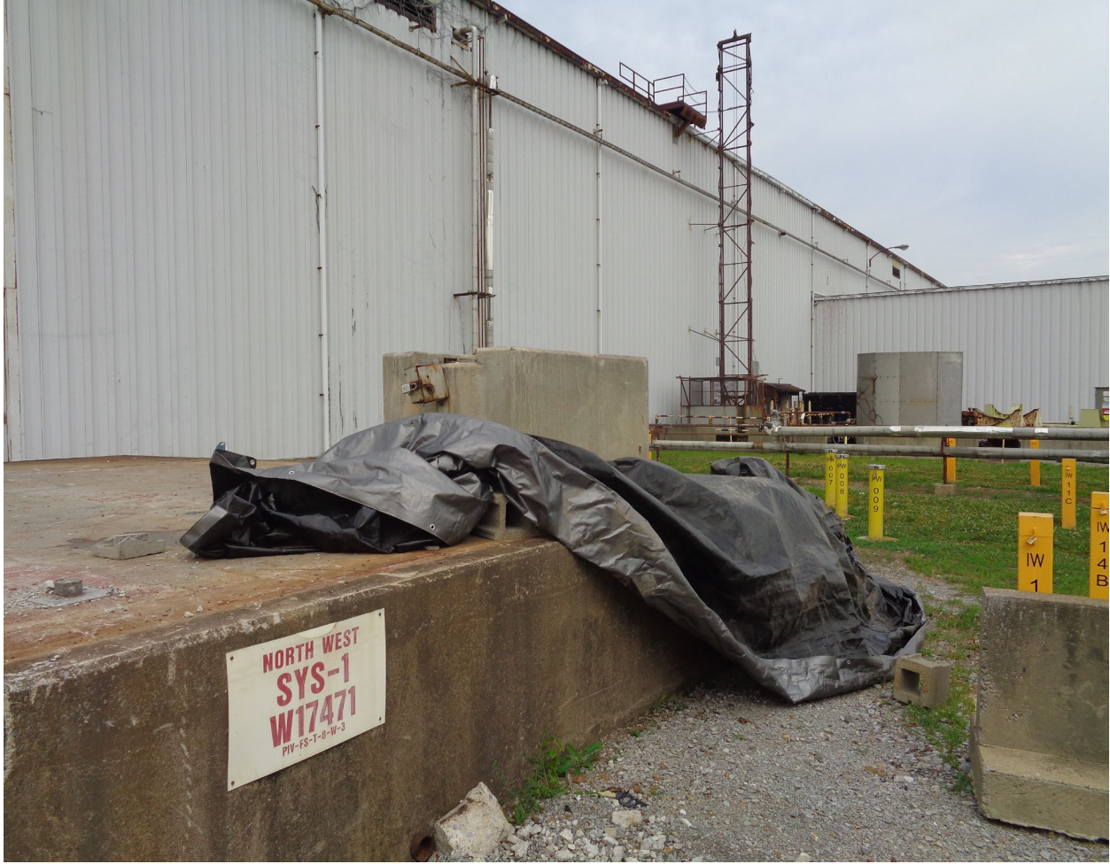
Figure 7. Concrete Structure Surrounding the Steel Cobalt Well on Remaining Slab Facing West
