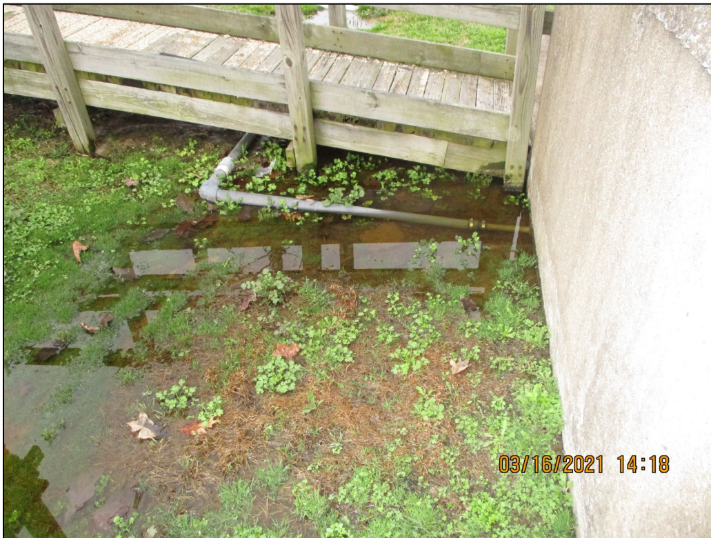
Figure 9. Standing Water in the Surface Ditch near the Sump Pump Discharge
