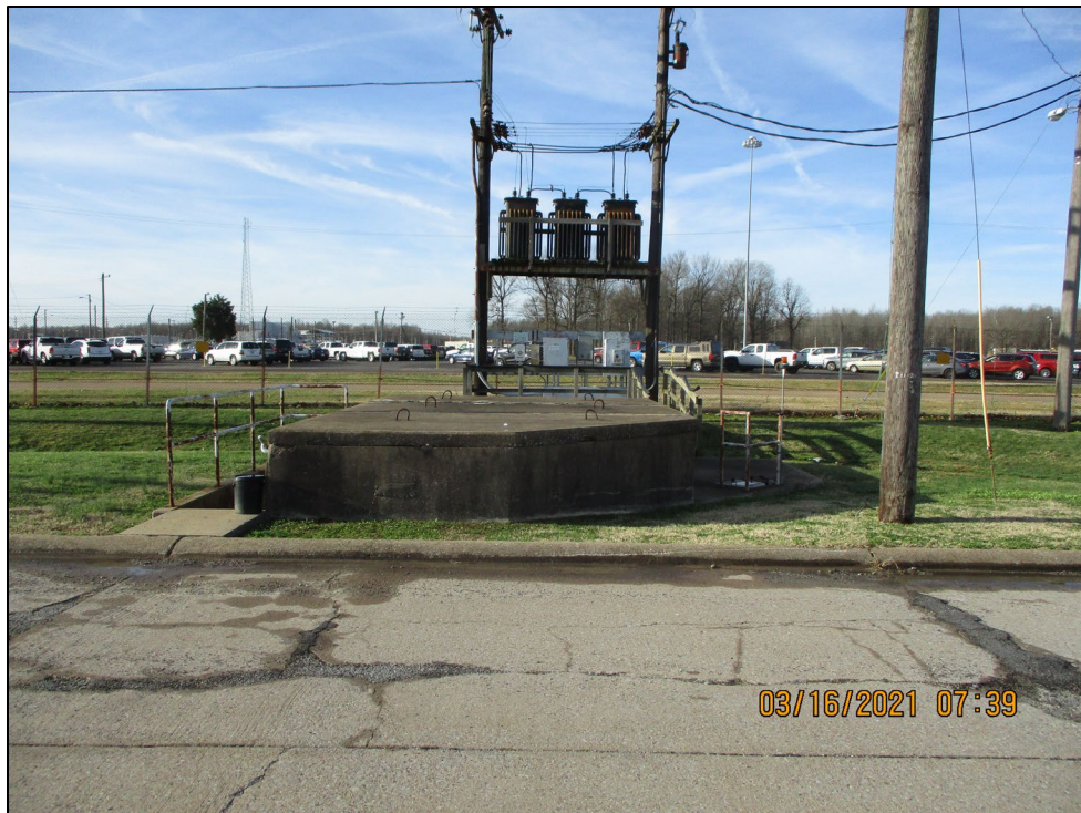
Figure 5. Exterior View of the C-611-T Booster Pump Station Plant Water (Looking South)
