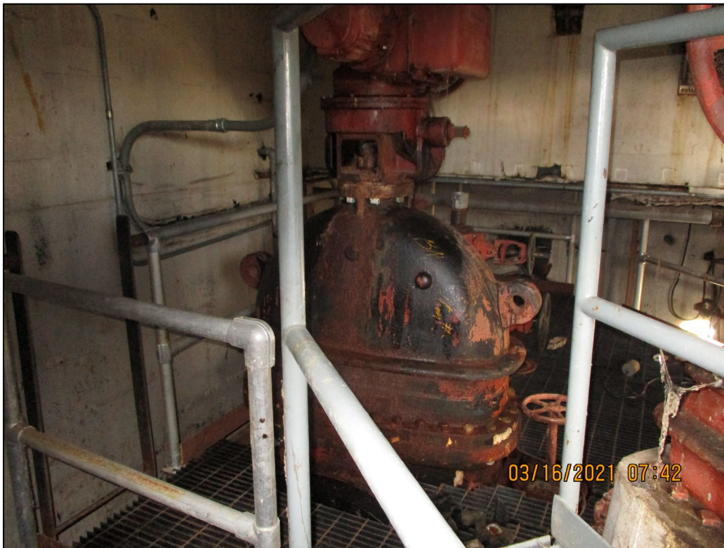
Figure 7. Interior View of C-611-T Showing the Plant Water Inlet Valve
