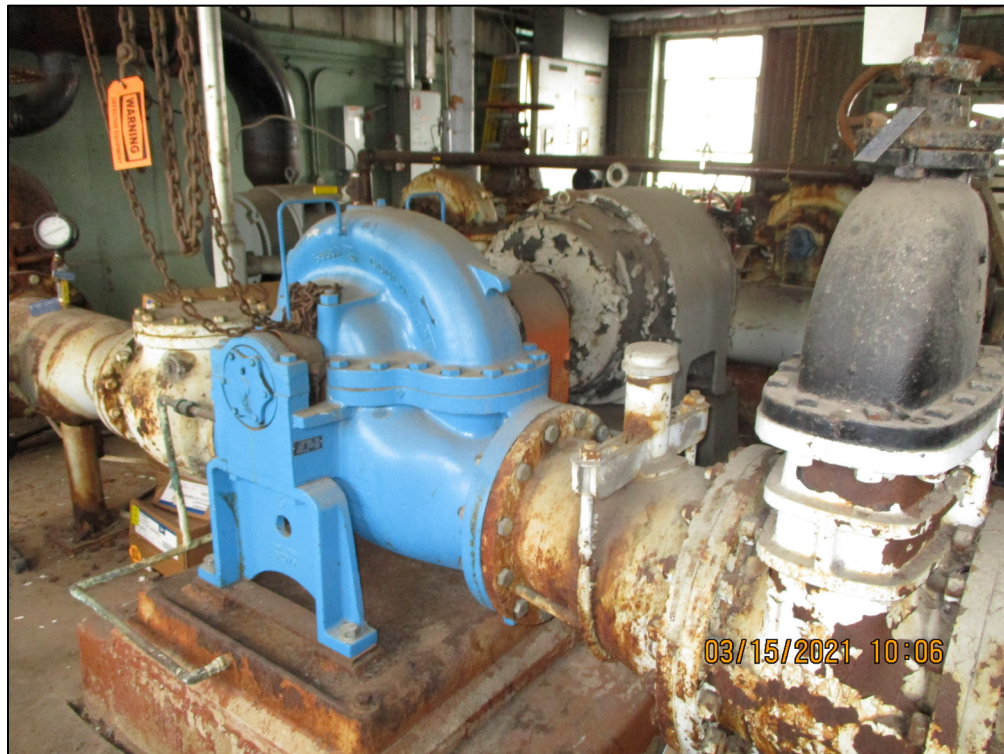
Figure 7. Interior View of C-611-P Looking Northeast Showing the No. 2 Booster Pump and Piping
