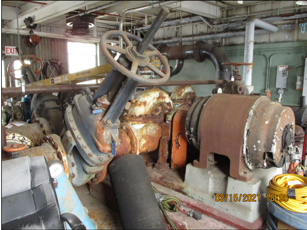
Figure 6. Interior View of C-611-P Showing the No. 1 Booster Pump and Motor
