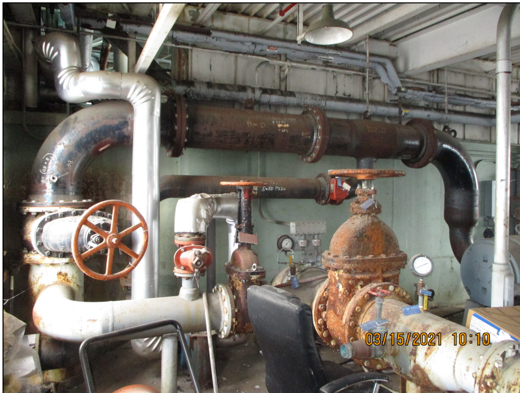
Figure 9. Piping and Valving Near the North Wall of the Building
