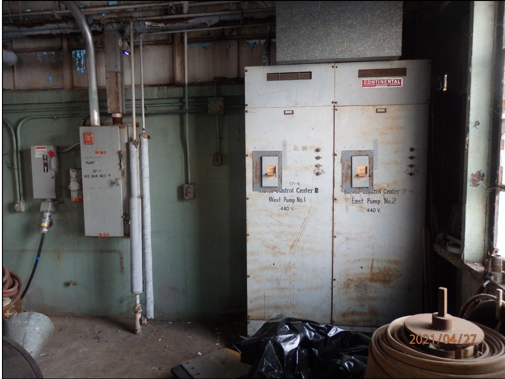
Figure 8. Electrical Switchgear for the Booster Pump Motors
