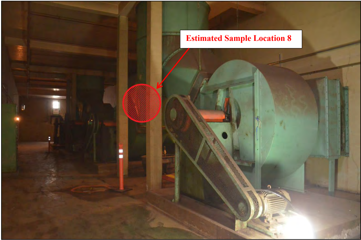
Figure D.8. Sample Location 8, Basement Fan Room Intake/Exhaust Plenum Fans 88/89
