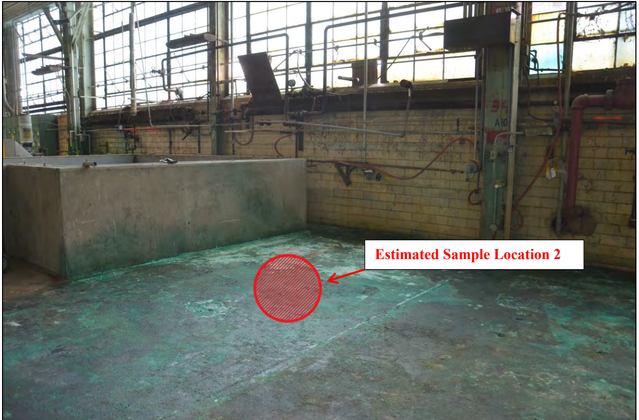
Figure D.2. Sample Location 2, Deteriorated Concrete near Column A10
