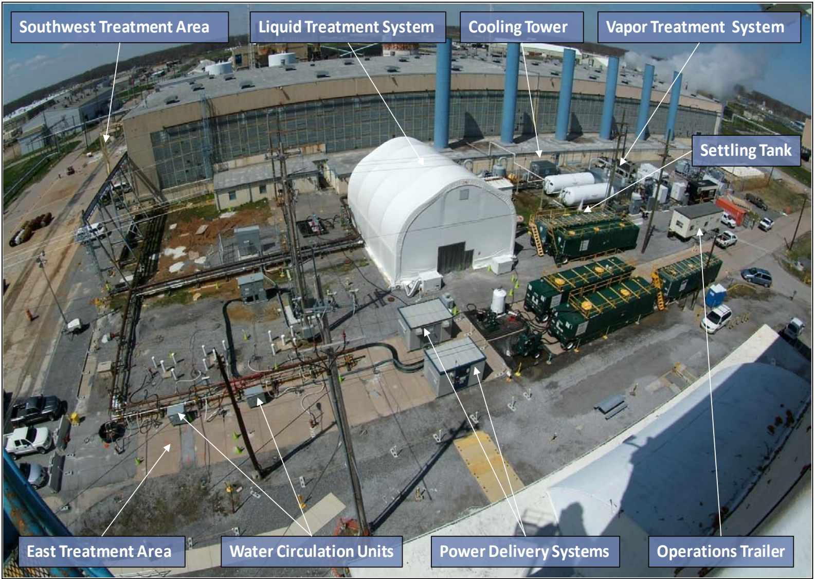
Figure 27. Picture of Groundwater/Vapor Treatment System Area
