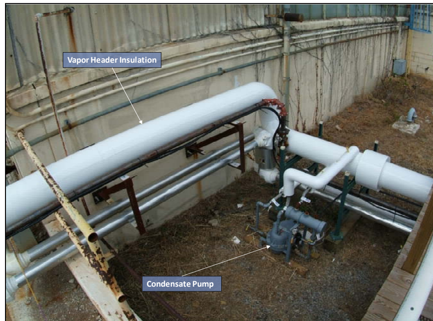
Figure 30. Condensate Pump and Insulated Vapor Header
