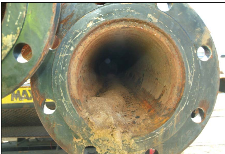
Figure 25. Sediment in the Vapor Extraction Header
