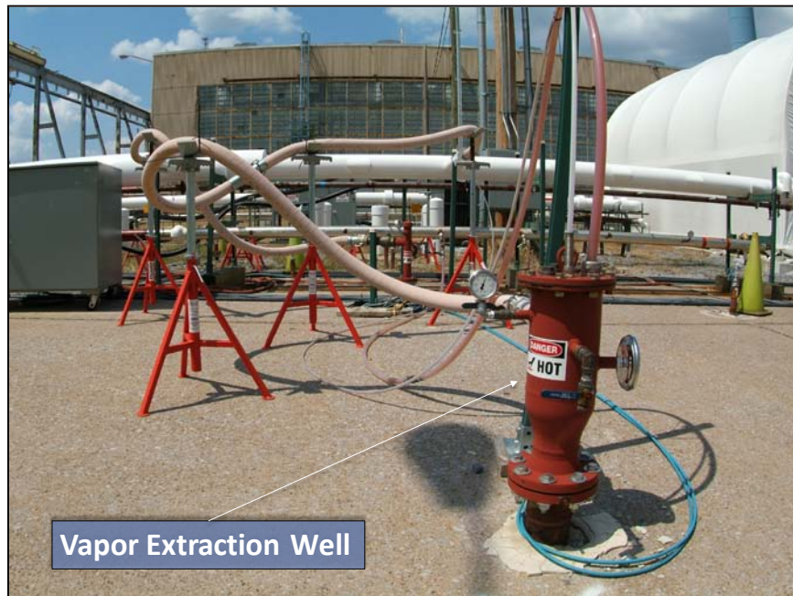
Figure 18. Vapor Extraction Well
