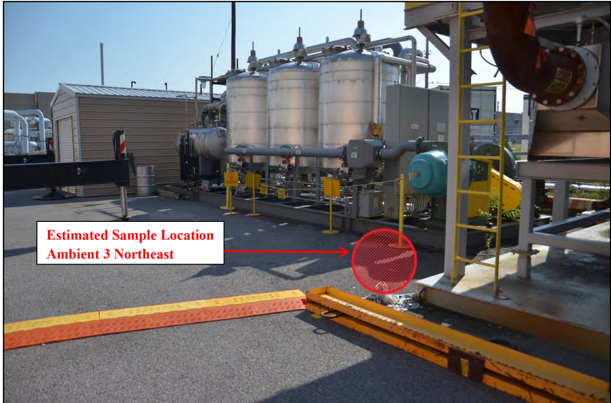
Figure D.11. Sample Location Ambient 3 Northeast, 87 ft East of Building, 54 ft North of Operation Stack
