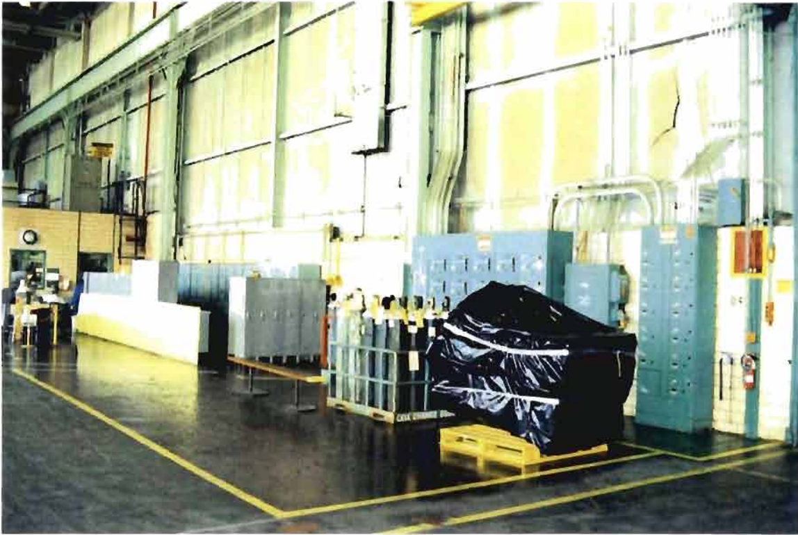
15. Diffusion Equipment and Scrap Removal Area - South
