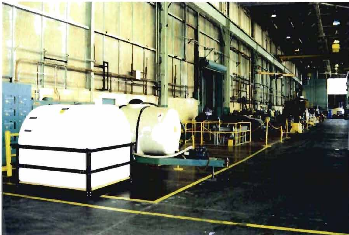
16. Diffusion Equipment and Scrap Removal Area - North
