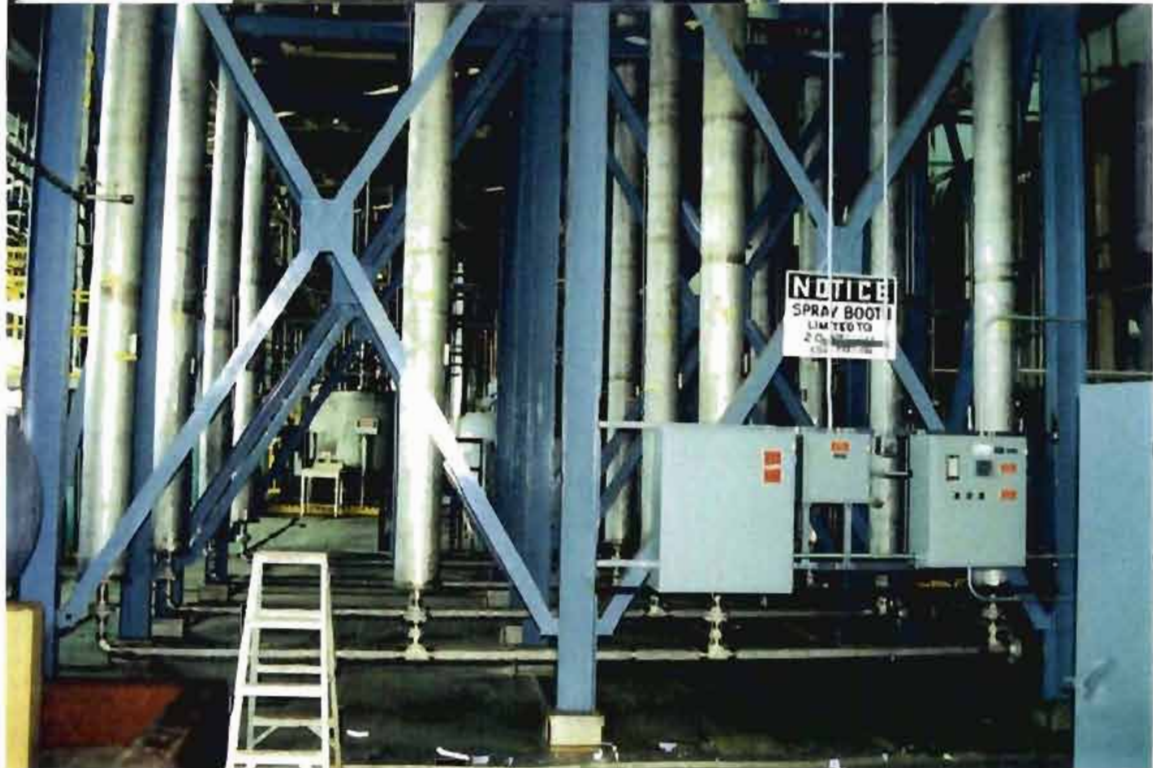
39. Spray Booth Tanks
