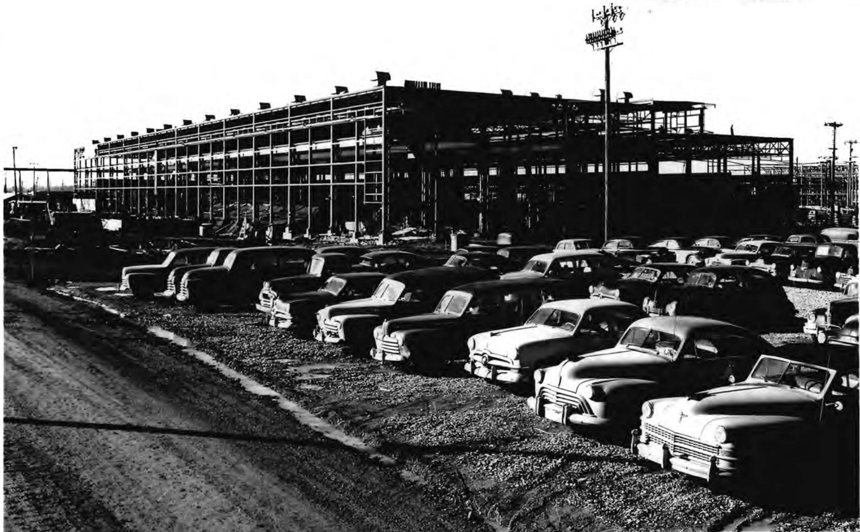
U.S. A.E.C. KENTUCKY AREA LOOKING SW TOWARD CLEANING BLDG C-400 F. H. MCGRAW & CO., CONTRACTOR AT-(15-1)-2 12-13-51
