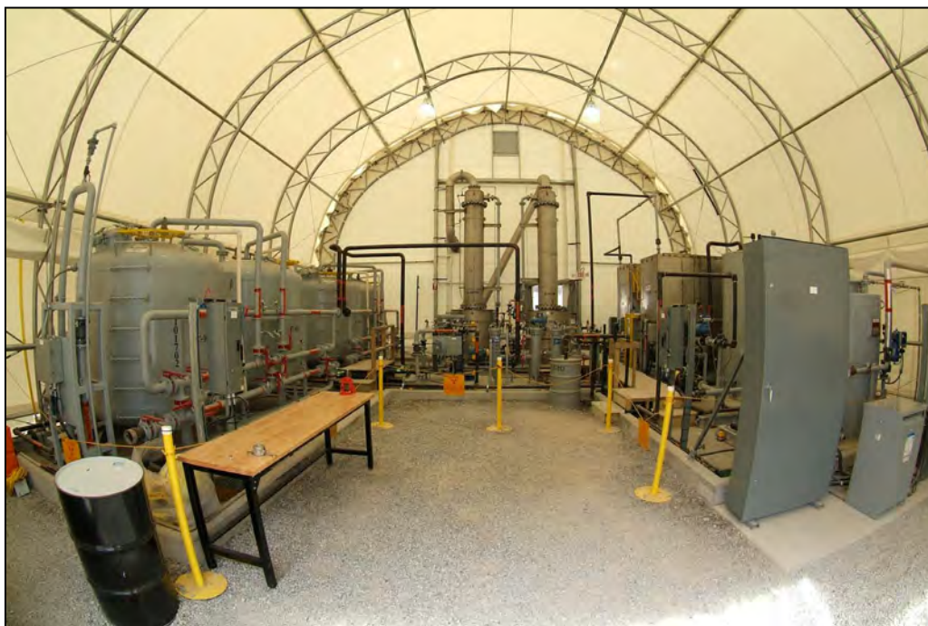
Figure 3.2. Treatment System for TCE-Contaminated Soil and Groundwater
