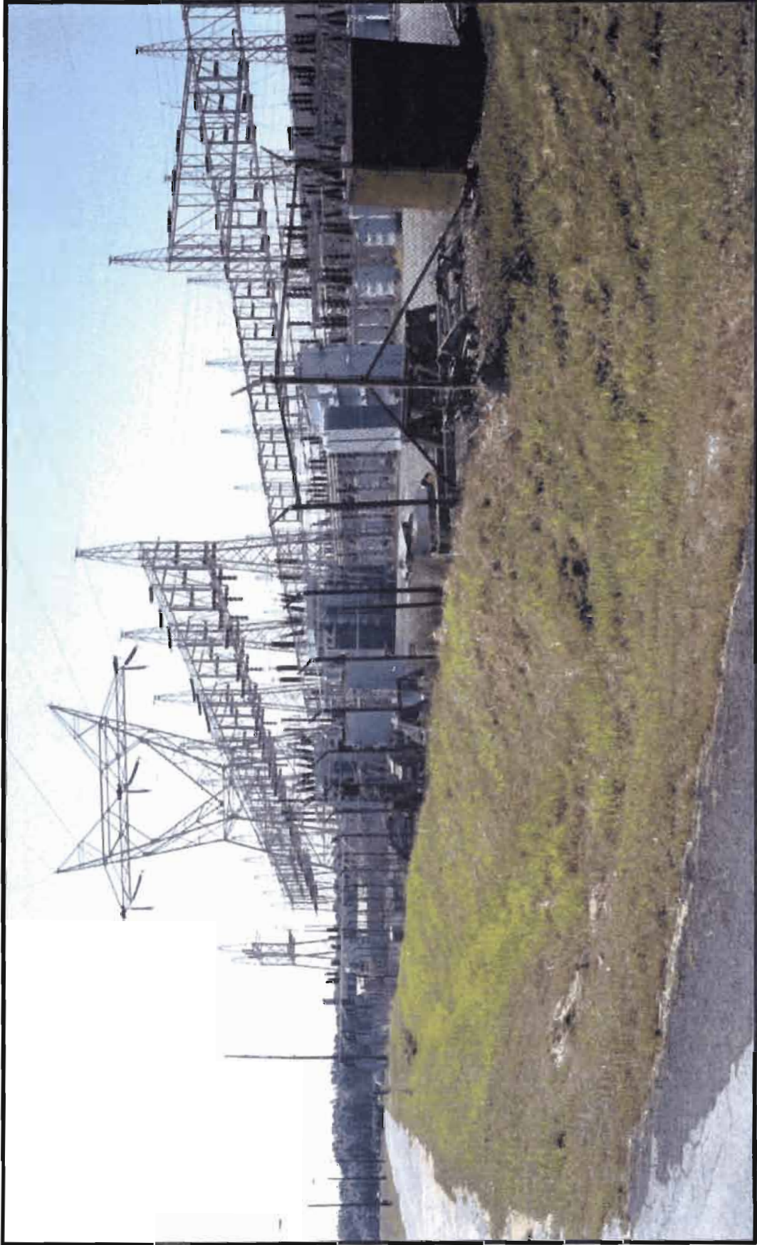
SWMU 85 -- North side of Electrical Switchyard C-537 looking east. DOE -- Paducah Gaseous Diffusion Plant. 1999.
