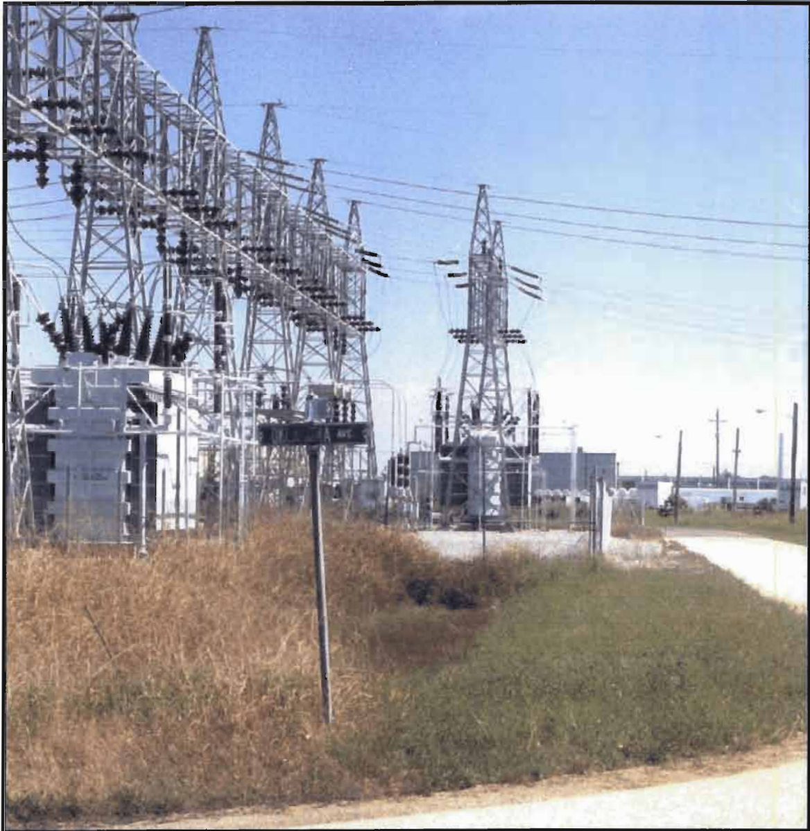
SWMU 82 – East side of Electrical Switchyard C-531 looking north. DOE – Paducah Gaseous Diffusion Plant, 1999
