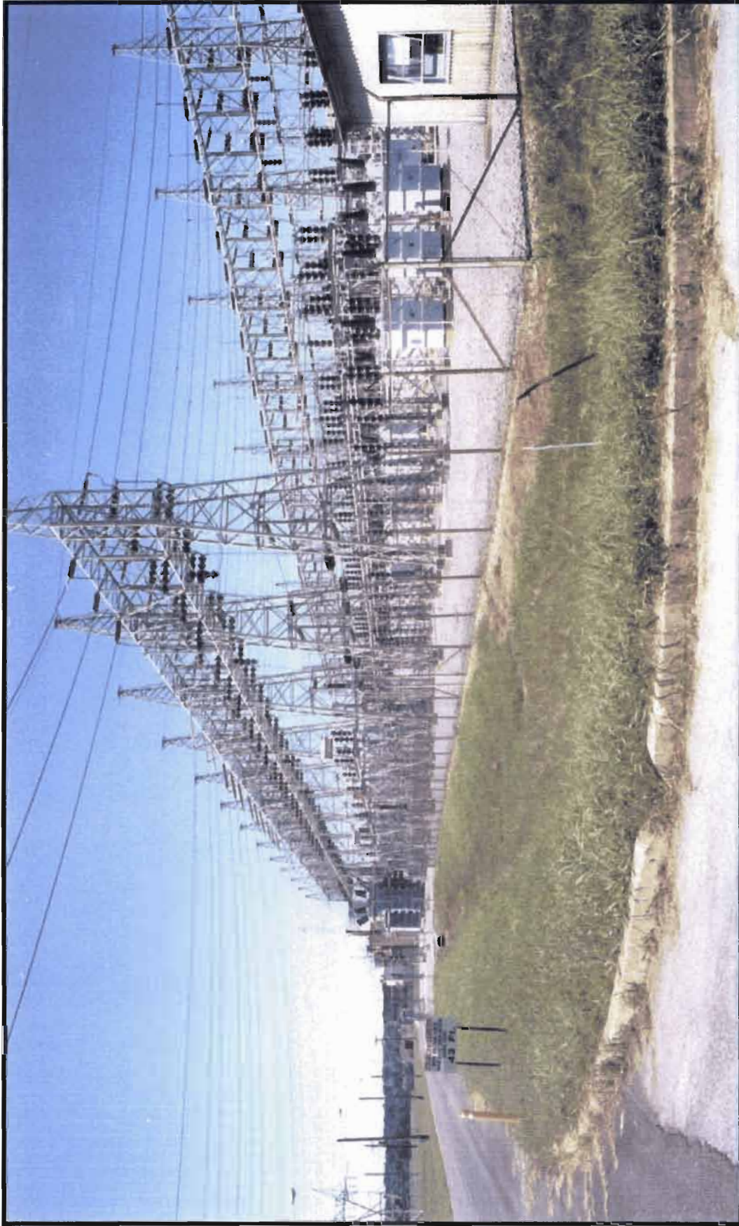
SWMU 83 – East side of Electrical Switchyard C-533 looking south. DOE – Paducah Gaseous Diffusion Plant. 1999.
