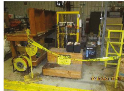
Battery Charging Station in Center Aisle
