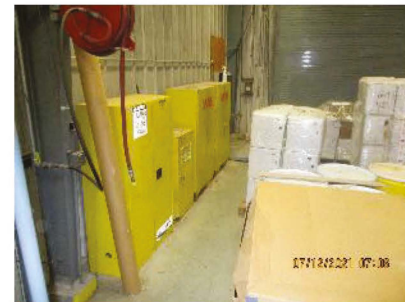
Flammable Items Storage Cabinet Along North Wall
