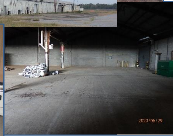
Removed light fixtures
