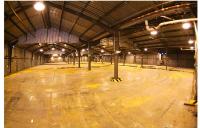
SWMU 144 - Metal pan area facing east C-746-A Hazardous and Mixed Waste Storage Facility February 14, 2011
