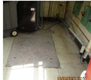
Electrical Manhole with Sump
