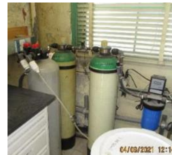
Deionized water system
