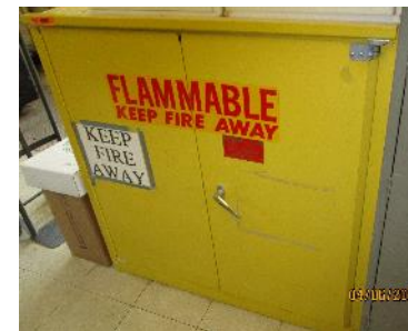
Flammable Cabinet - Contains wasp spray, hornet spray and other types of aerosol sprays
