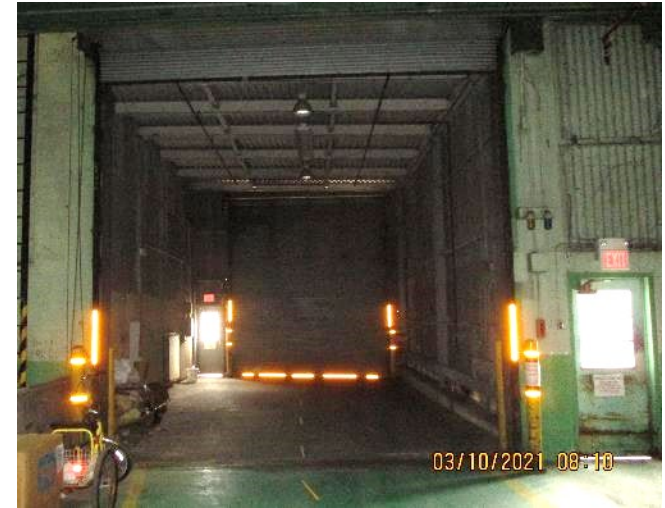
Looking east into the C-720-J Air Lock from inside C-720
