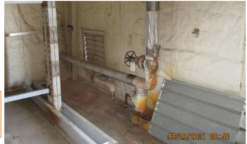
Steam and Condensate Piping in Northwest Corner of C-720-H
