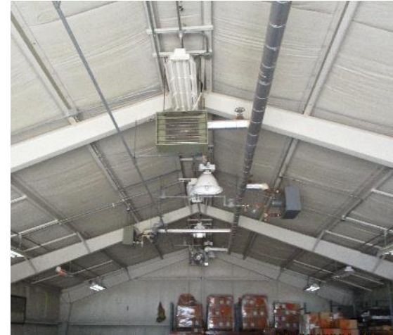
Ceiling View Showing Heaters/ Lighting
