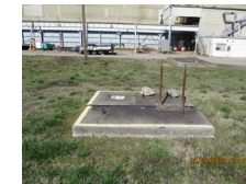
H-Loop Return Bypass to Blending Tower Vault
