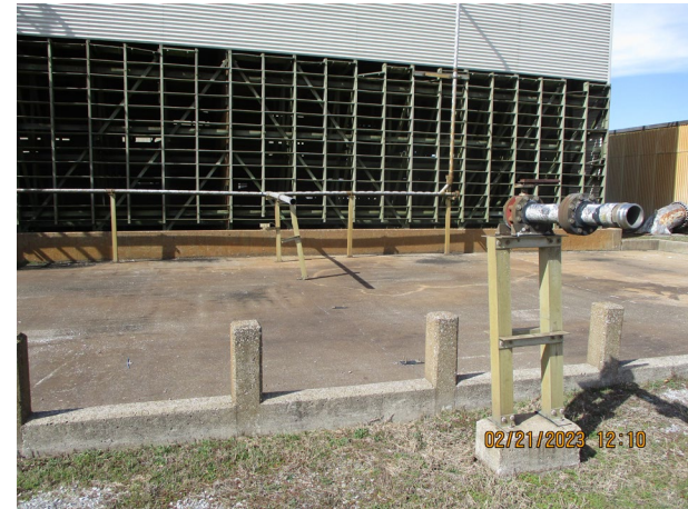
C-637-4 Southeast Corner – Lateral and Flush Lines
