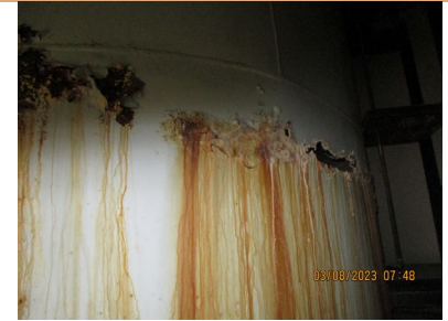
C-637-6 - Permutit® Sand Filter Tank (Corrosion Damage)
