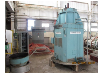
C-637-1 - Center Structure Electric RCW Pump Motor
