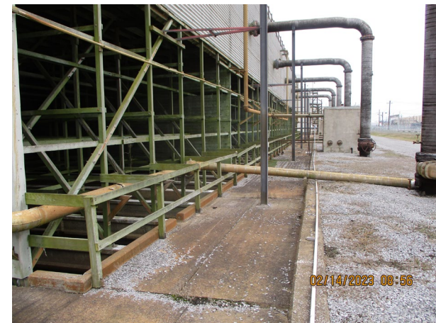
West Side Risers
