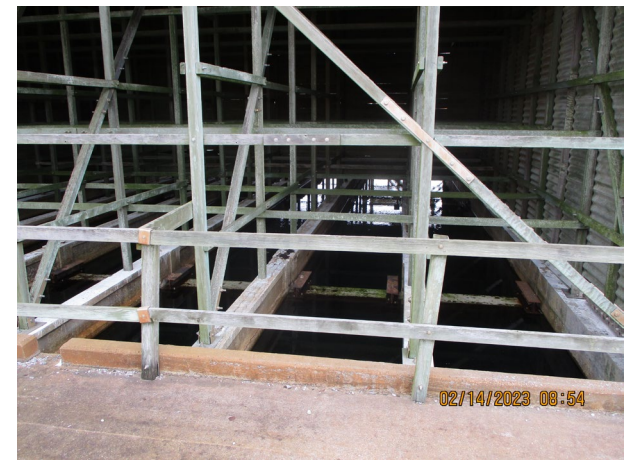
C-637-2A Cooling Tower – Basin
