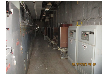
C-637-1 – East Wing Switchgear Room – Looking South
