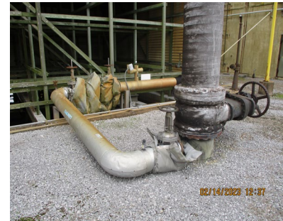
C-637-2B Cooling Tower Northeast Plume Pump and Treat Line to Riser No. 1
