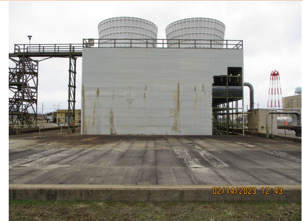
C-637-2B Cooling Tower – North Side
