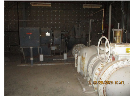
C-637-3 - Skid Frame with Blend Motor and Pump
