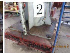
C-637-1 - Center Structure Pump Oil Stain
