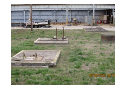
Instrument Connection Vault (Round Vault in Background)
