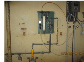
C-637-1 - West Wing Chlorine Rotameter
