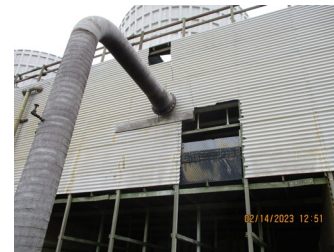
C-637-2B – Structural Damage near Riser No. 4
