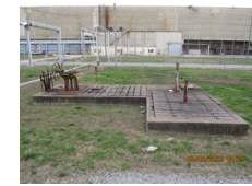
G-Loop Supply/G-Loop Supply Crossover Vault
