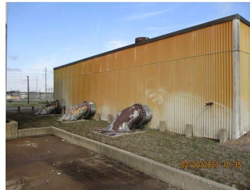
C-637-3 - Pump Suction Lines Exterior View
