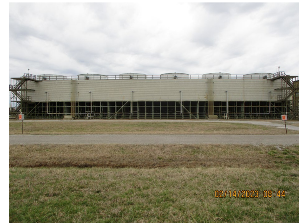
C-637-2A Cooling Tower – East Side
