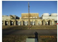
External Electrical Transformers
