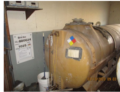
C-637-1 - West Wing Calgon Area
