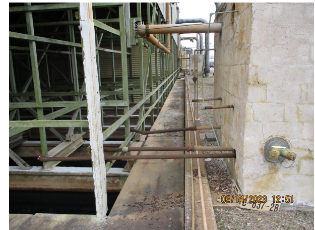
C-637-2B Cooling Tower –West Side (Area between Basin and Fire Sprinkler Houses)
