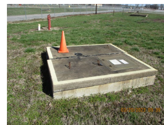
G-Loop Return Blending Tower Crossover Vault
