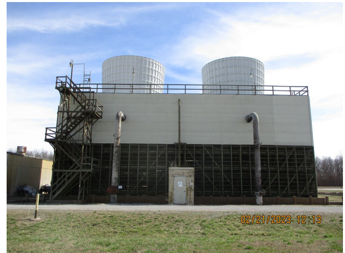
C-637-4 Blending Cooling Tower – West Side
