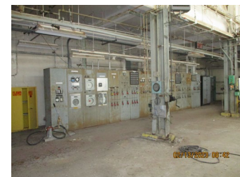
C-637-1 - Center Structure Control Panel
