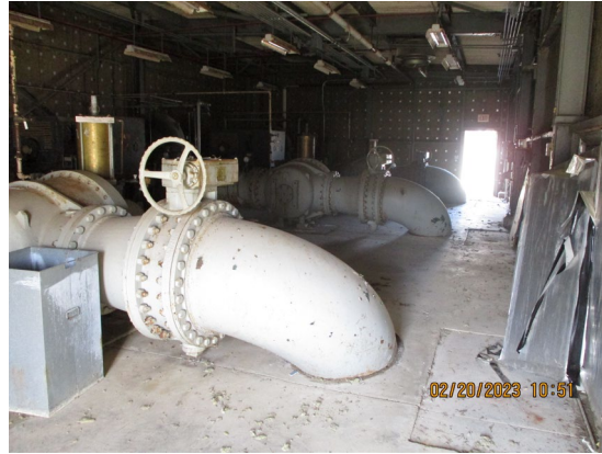
C-637-3 - Pump Discharge Lines
