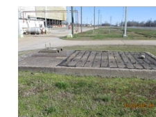
H-Loop Supply Venturi Vault
