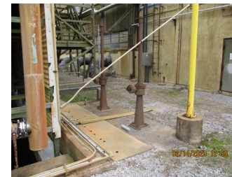
C-637-2B – Flume Sluice Gates
