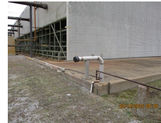
C-637-2A – Fire Protection Connection Point
