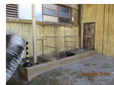
Wet Well Overflow/Blowdown Vault
