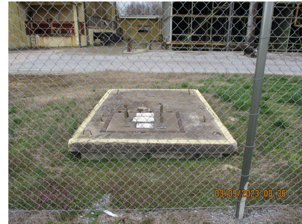
H-Loop Return to Blending Tower Vault
