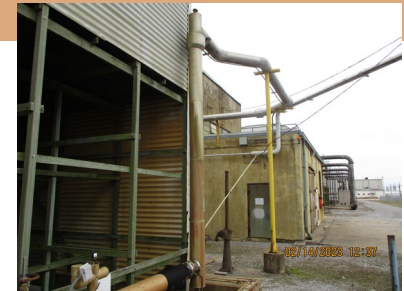
C-637-2B – Cooling Tower Northeast Plume Pump and Treat Lines (Air-gapped)
