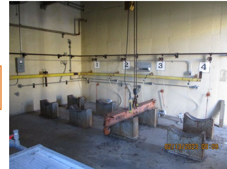
C-637-1 - West Wing Chlorine Feed Header
