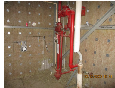
C-637-3 - Fire Sprinkler System
