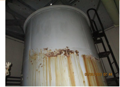
C-637-6 – Permutit® Sand Filter Tank
