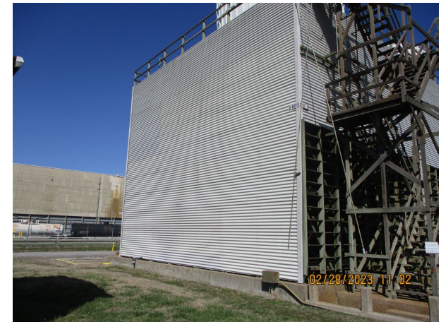
C-637-5 Blending Cooling Tower - South Side
