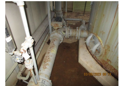
C-637-6 – Flow Orifice and Discharge Piping
