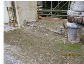
C-637-2B– RCW Hot Water Supply to Fire House Heater
