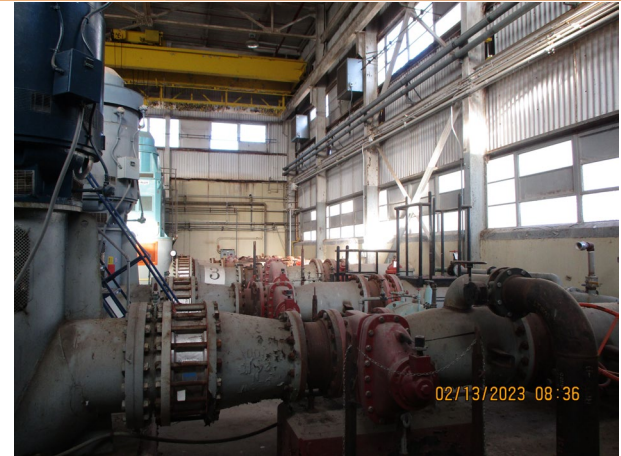
C-637-1 - Center Wing RCW Pumps and Discharge Lines
