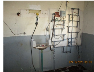
C-637-1 - West Wing Eye Wash and Corrosion Test Loop
