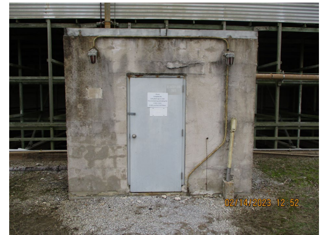
C-637-2B Sprinkler System - External View
