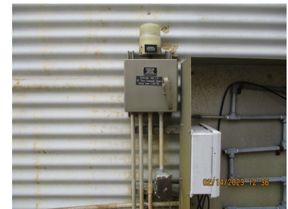
C-637-2B – Cooling Tower Northeast Plume Pump and Treat Terminal Box
