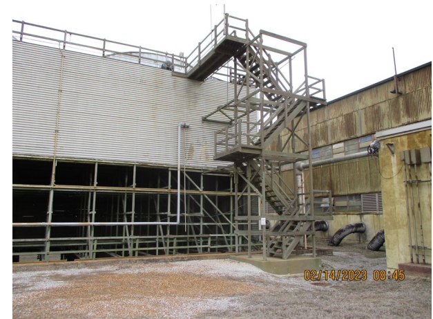
C-637-2A Cooling Tower – Northeast Corner
