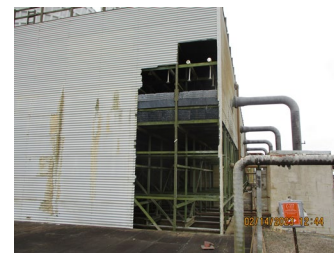
C-637-2B–Interior and Exterior Structural Damage
