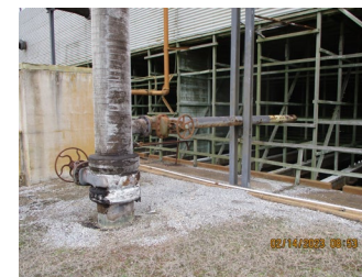
C-637-2A – Riser No. 1 and Bypass Line
