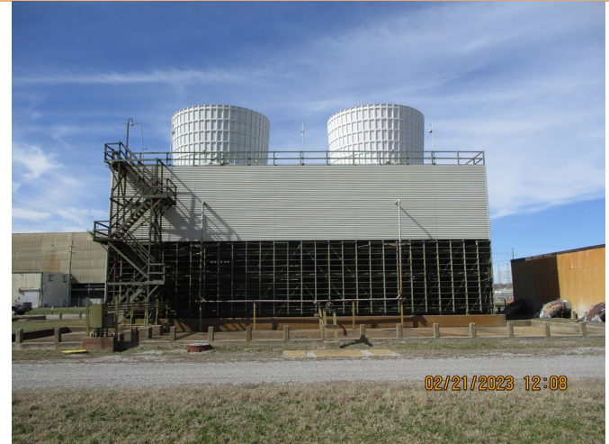
C-637-4 Blending Cooling Tower – East Side
