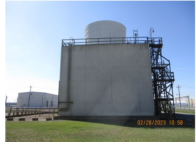
C-637-5 Blending Cooling Tower – North Side
