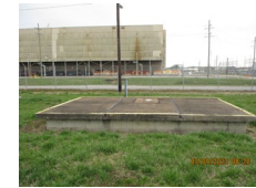
G-Loop Return Bypass Vault
