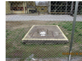
H-Loop Return to Blending Tower Vault
