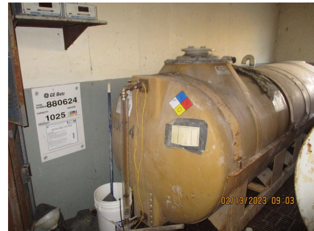
C-637-1 West Wing Betz Chemical Feed Tank
