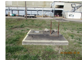
H-Loop Return Bypass to Blending Tower Vault
