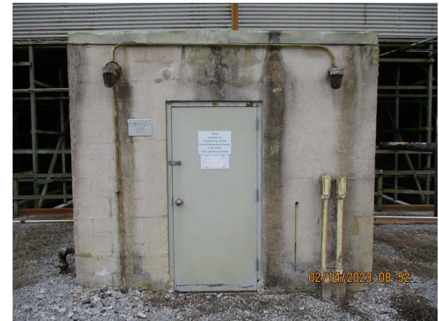
C-637-2A Sprinkler System - External View
