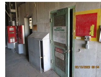
C-637-1 – East Wing Battery Room Charger Entrance
