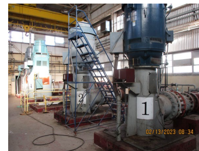
C-637-1 – Center Structure RCW Pump #1
