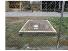
H-Loop Return to Blending Tower Vault
