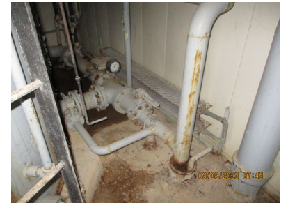
C-637-6 – Piping System (East Wall)
