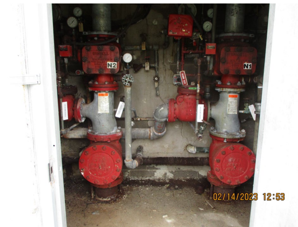
C-637-2B Sprinkler System - Internal View
