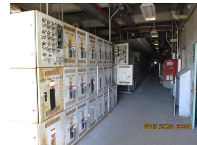
C-637-1 - East Wing Interior Switchgear Room
