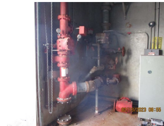
C-637-1 - East Wing Transformer Sprinkler System
