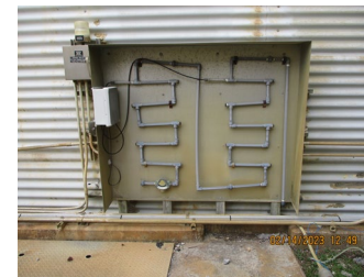
C-637-2B–Corrosion Testing Area
