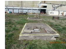
H-Loop Return Bypass Vault
