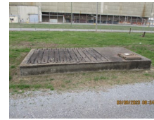
G-Loop Supply Venturi Vault
