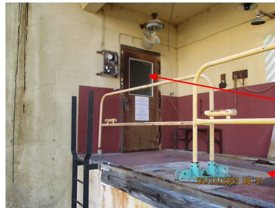
C-637-1 West Wing Sulfuric Acid Pig and Tanks Location
