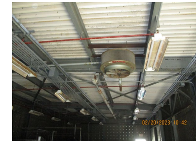
C-637-3 – Steam Heater
