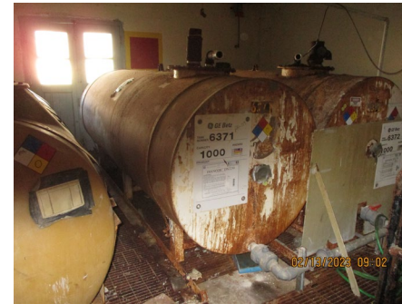
C-637-1 - West Wing Calgon Room (Corrosion Inhibitor Feed Area)
