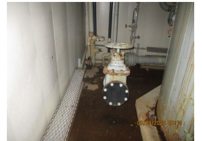
C-637-6 -Sanitary Water Line (Capped)
