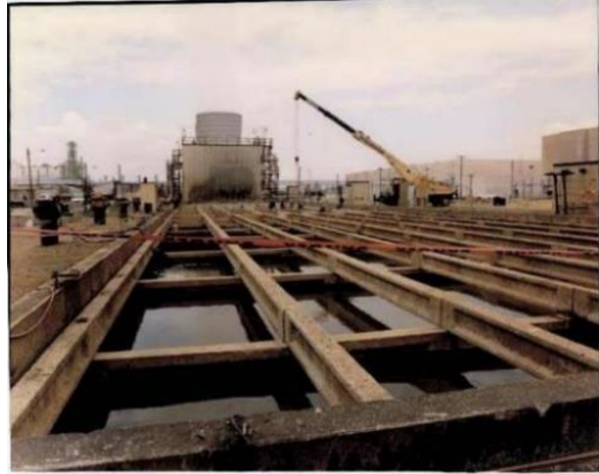
Historical photo of main cooling tower replacement project (Photo of C-637 Main Cooling Tower)
