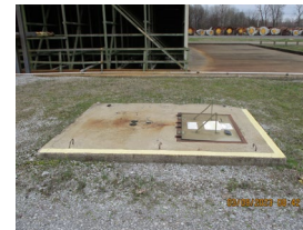
H-Loop Return to Blending Tower Crossover Vault
