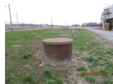
Instrument Connection Vault
