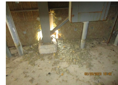
C-637-3 – Damaged Insulation
