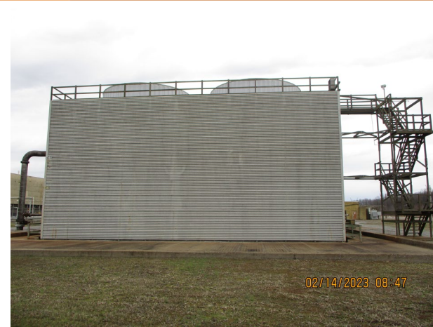
C-637-2A Cooling Tower – South Side
