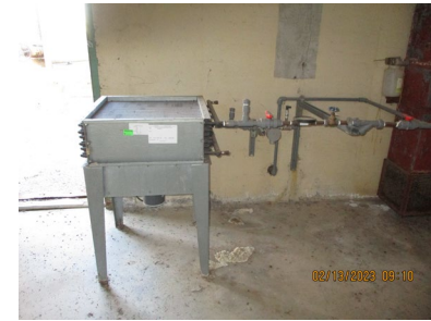
C-637-1 - West Wing Chlorine Monitor Cooler
