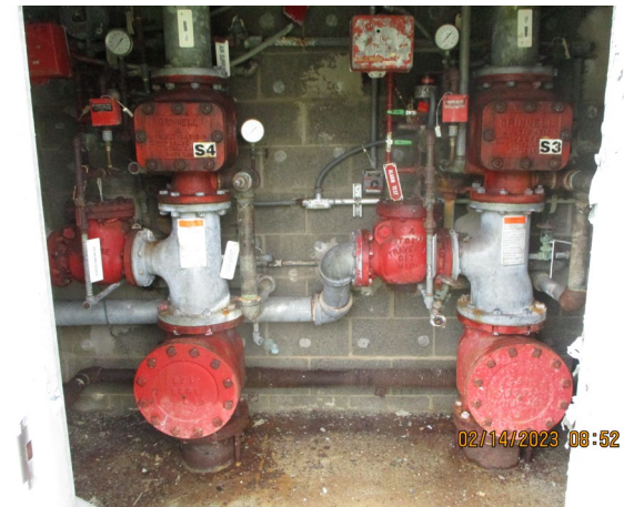
C-637-2A Sprinkler System - Internal View
