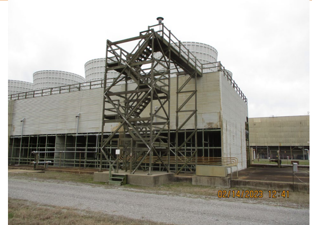
C-637-2B Cooling Tower – Northeast Side
