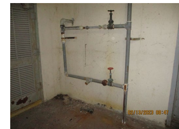
C-637-1 - East Wing Sanitary Water Supply
