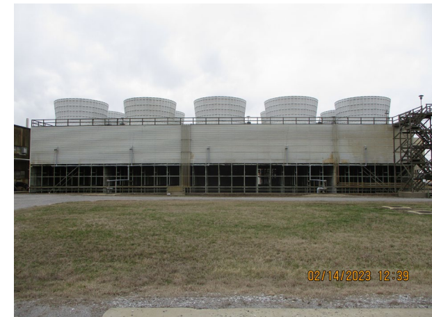
C-637-2B Cooling Tower – East Side
