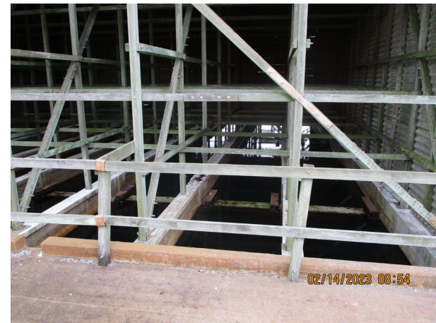
C-637-2A Cooling Tower – Interior View
