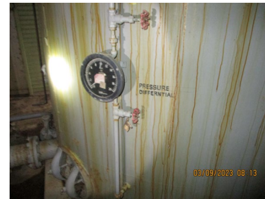
C-637-6 -Permutit® Sand Filter Tank (Pressure Differential Indicator)
