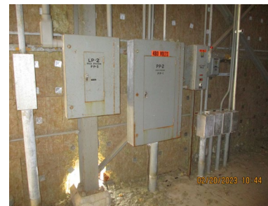
C-637-3 – Electrical Panels
