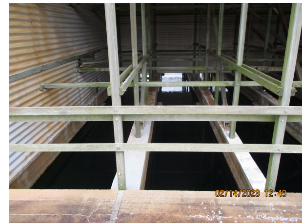
C-637-2B Cooling Tower – Interior View
