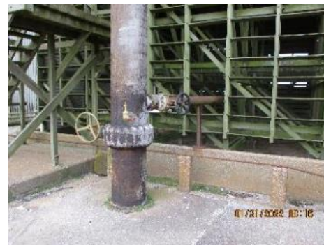
C-635-4 – No. 9 Riser Block Valve and Hot Water Bypass Line
