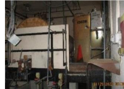
C-635-1 - West Wing Calgon Room (Corrosion Inhibitor Feed Area)
