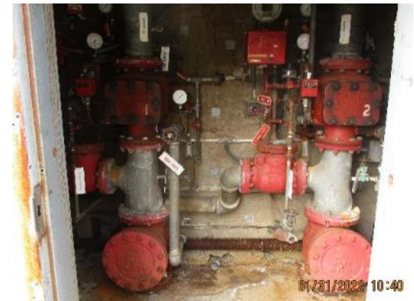
C-635-2 Sprinkler System - Internal View
