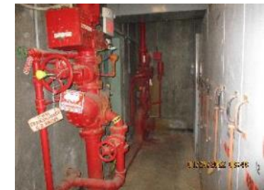
C-635-1 - East Wing Transformer Sprinkler System
