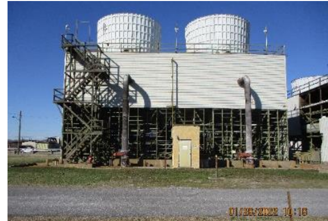
C-635-5 Blending Cooling Tower – East Side
