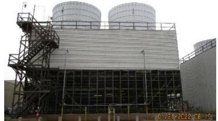
C-635-4 Blending Cooling Tower – West Side
