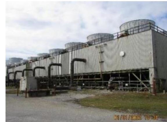
C-635-2 Cooling Tower – East Side
