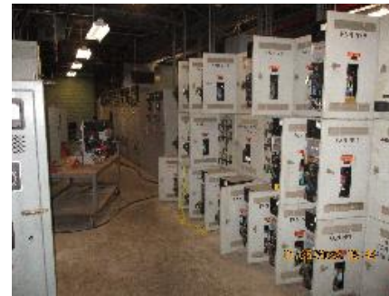
C-635-1 - East Wing Switchgear Room – Looking North
