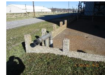
C-635-5 - Southwest Corner Water Withdrawal for Firefighting
