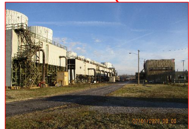
C-635 Cooling Tower Photo: 2/2022
