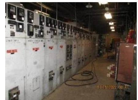
C-635-1 - East Wing Switchgear Room
