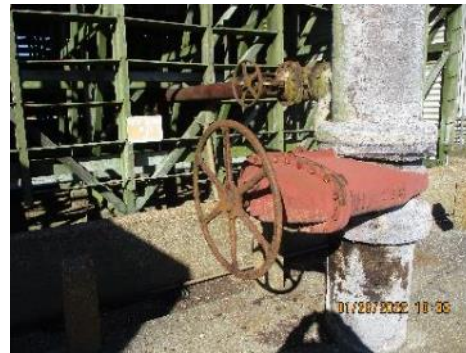
C-635-5 – No. 11 Riser Block Valve and Hot Water Bypass Line
