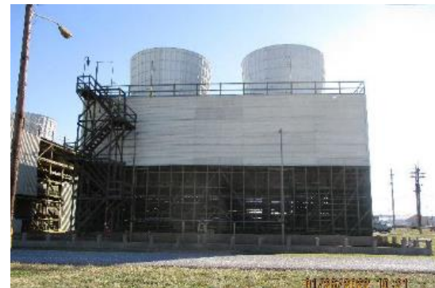
C-635-5 Blending Cooling Tower - West Side
