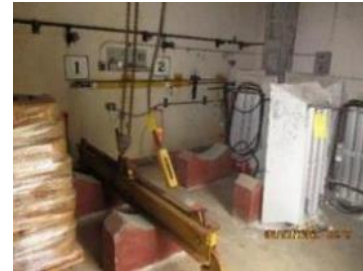
C-635-1 - West Wing Chlorine Area (with soda ash and Cal-Rod heaters)
