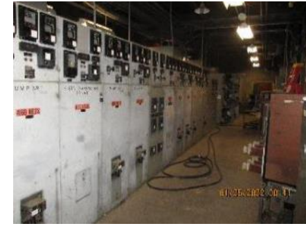
C-635-1 - East Wing Switchgear Room – Looking South
