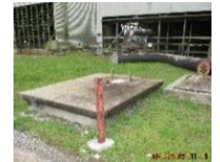
E-Loop Return to Blending Tower Vault
