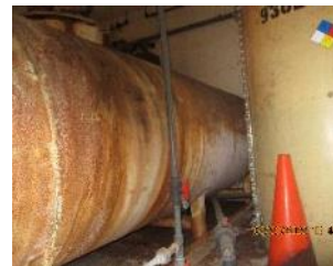
C-635-1 - West Wing Chlorine Tank
