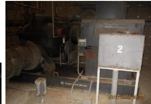
C-635-3 - Skid Frame with Blend Motor and Pump
