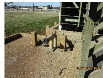
C-635-5 - Southeast Corner Water Withdrawal for Firefighting
