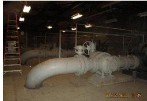
C-635-3 - Pump Discharge Line
