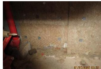
C-635-3 - Damaged Wall Insulation
