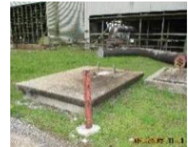
E-Loop Return Vault to C-635-5 Blending Tower
