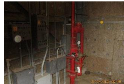
C-635-3 - Fire Sprinkler System
