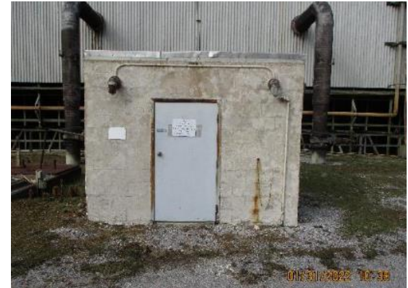
C-635-2 Sprinkler System - External View
