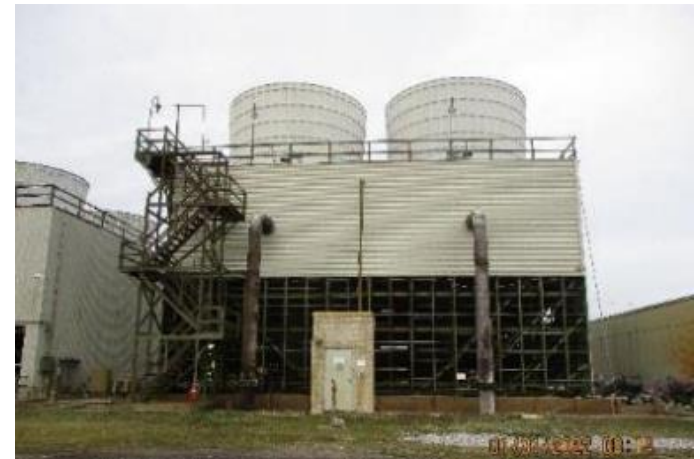
C-635-4 Blending Cooling Tower – East Side
