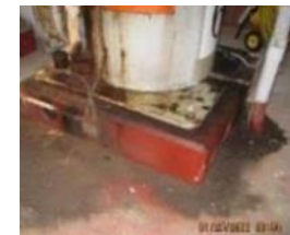
C-635-1 - Center Structure Pump Oil Stain
