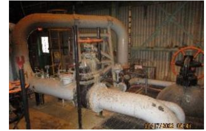
C-635-1 - Center Structure Surge Relief Valve
