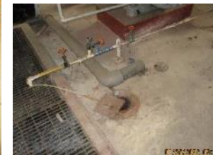
Gray pipe from chemical area feeding into to wet well
