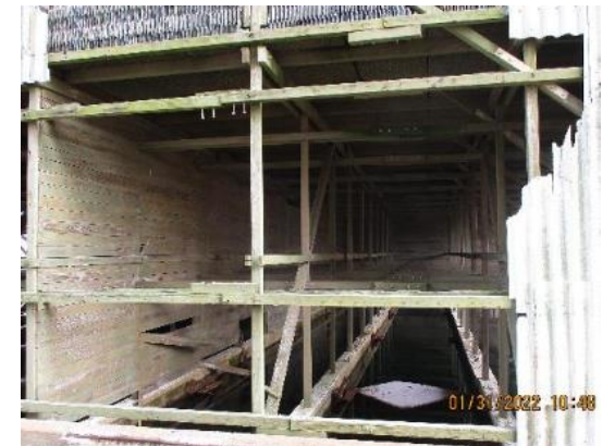
C-635-2 Cooling Tower – Interior View
