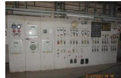
C-635-1 - Center Structure Control Panel
