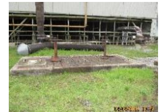
F-Loop Return and Bypass Vault (Valve Vault B)
