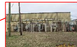
External Electrical Transformers
