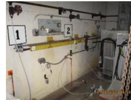
C-635-1 - West Wing Chlorine Feed Header
