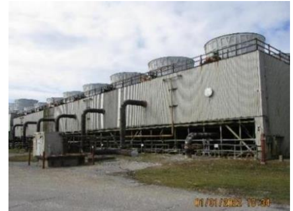
C-635-2 Cooling Tower – East Side
