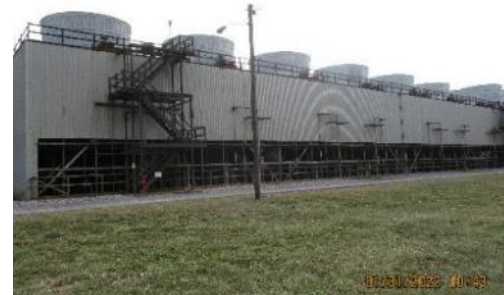
C-635-2 Cooling Tower – West Side
