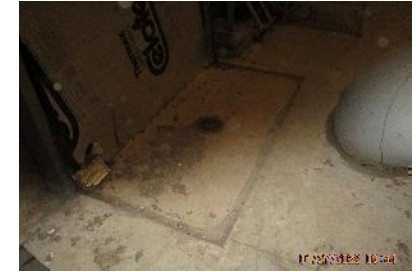
C-635-3 - Floor Drains
