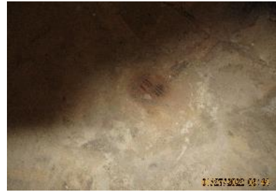
C-635-3 - Floor Drains
