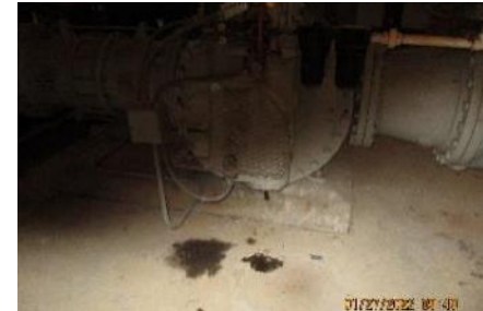
C-635-3 - Oil Staining
