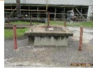
F-Loop Return to Blending Tower Vault
