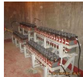
C-635-1 - East Wing Lead Calcium Batteries
