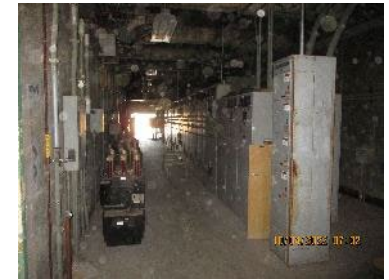
C-633-1 – East Wing Switchgear Room – Looking North
