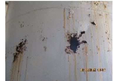
C-633-6 - Permutit® Sand Filter Tank (Corrosion Damage)
