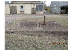
Hot Water Bypass Vault
