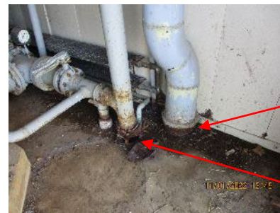
C-633-6 – Drain Lines to Storm Sewer and C-633-2B Basin
