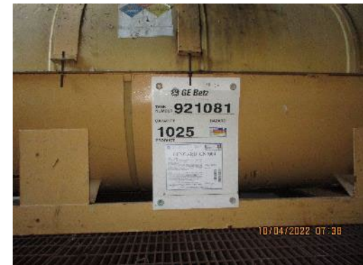
C-633-1 West Wing Betz Chemical Feed Tank
