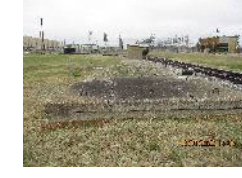
Plant Water Valves (Makeup Water) Vault
