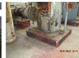
C-633-1 - Center Structure Pump Oil Stain
