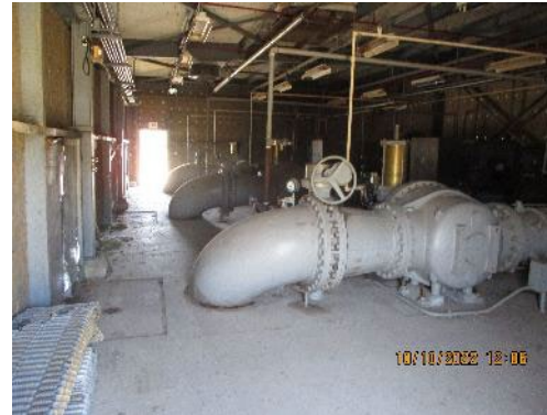
C-633-3 - Pump Discharge Lines
