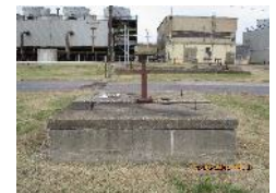
C-Loop Return Bypass to Blending Tower Vault
