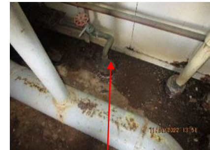
C-633-6 – RCW Line for Fin Heating - Drain Line to C-633-2B Basin
