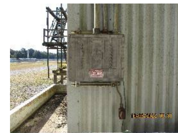
C-633-2A – Light Switch Panel to Tower and Fire Houses
