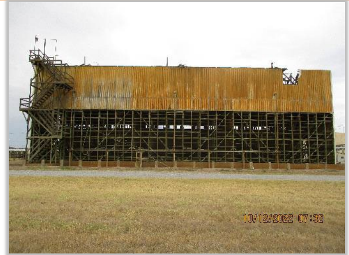
C-633-4 Blending Cooling Tower – East Side
