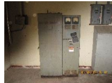
C-633-1 – East Wing Battery Charger
