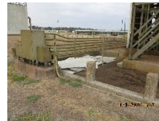
C-633-4 Electric Conduit and Cooling Tower Siding
