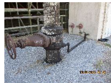
C-633-2A – Riser No. 7 with Hot Water Line to Fire House Heaters
