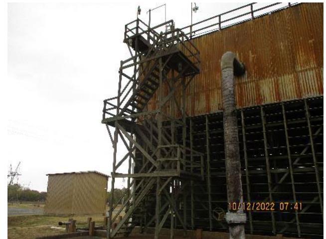
C-633-4 West Side – Riser No. 11
