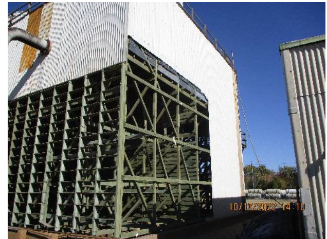
C-633-5 Blending Cooling Tower - South Side
