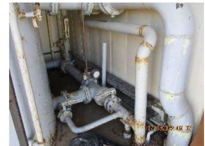
C-633-6 – Piping System (West Wall)
