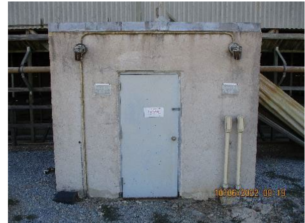
C-633-2A Sprinkler System - External View
