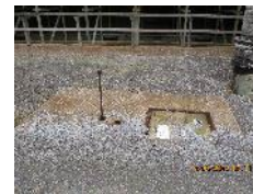
C-Loop Return Blending Tower Crossover Vault
