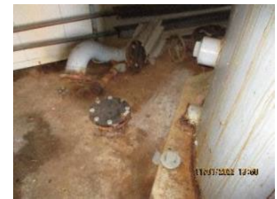
C-633-6 -Sanitary Water Line (Capped at Floor)
