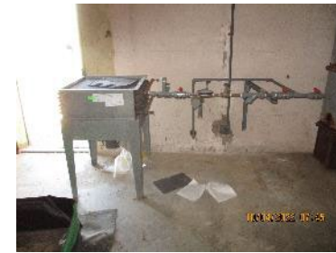
C-633-1 - West Wing Chlorine Monitor Cooler
