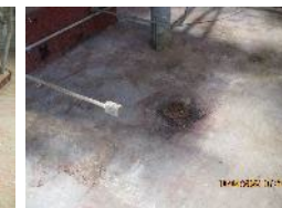
C-633-1 - Center Structure Typical Floor Drain (damaged around edge)
