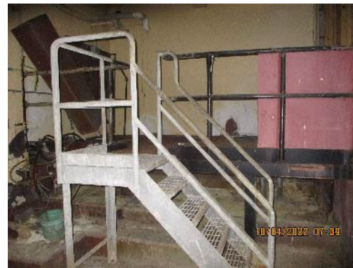
C-633-1 West Wing Sulfuric Acid Pig and Tanks Location
