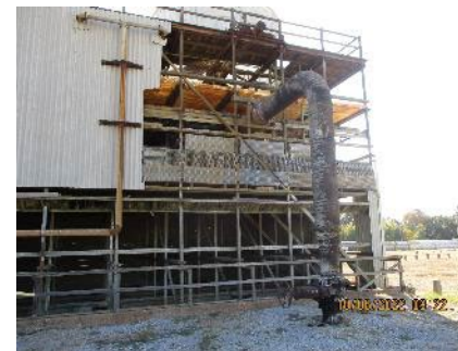
C-633-2A – Southwest Corner Structural Damage
