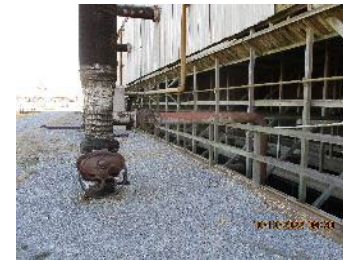
C-633-2B— Riser No. 1 and Bypass
