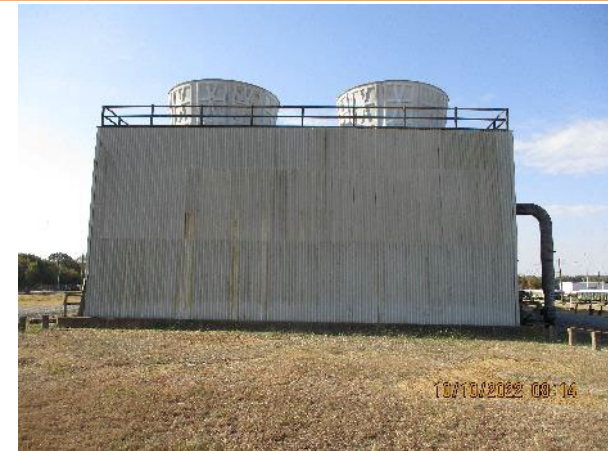
C-633-2B Cooling Tower – North Side
