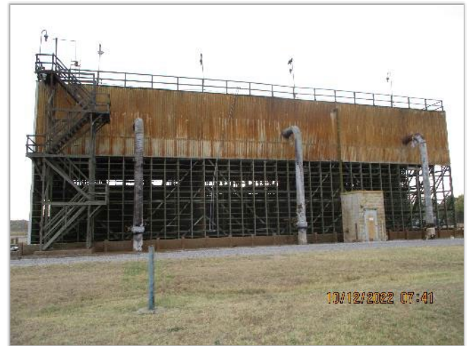
C-633-4 Blending Cooling Tower – West Side
