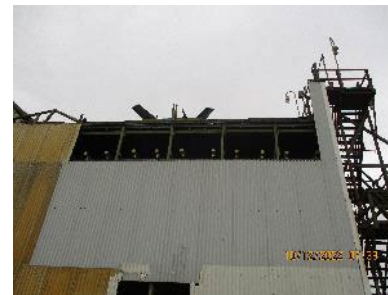
C-633-4 – North Side (Structural Top Damage – Missing Shrouds)
