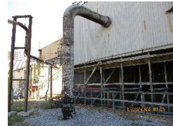
C-633-2A – Riser No. 8 with Bypass
