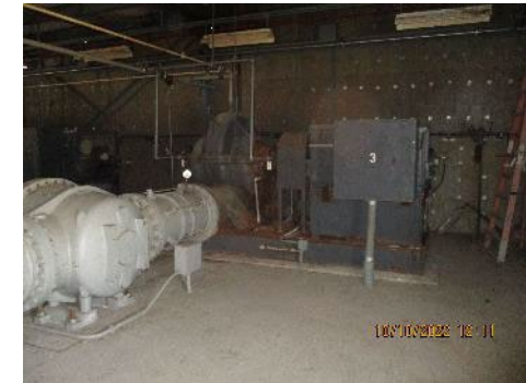
C-633-3 - Skid Frame with Blend Motor and Pump
