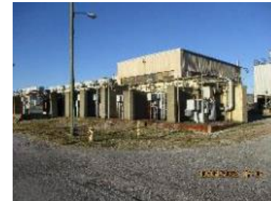
C-633-1 - East Wing External Transformers
