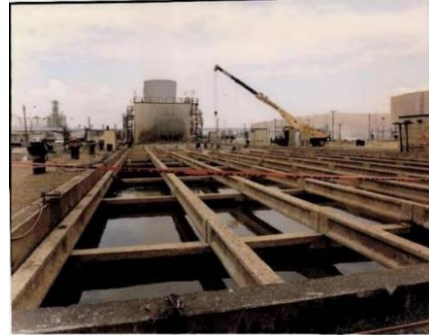
Historical photo of main cooling tower replacement project (Photo of C-633 Main Cooling Tower)
