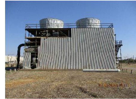
C-633-2A Cooling Tower South Side Structural Damage
