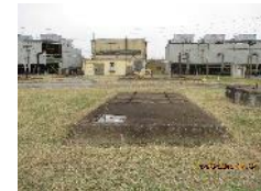
D-Loop Supply Venturi Vault
