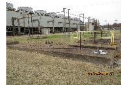
D-Loop Supply Crossover/D-Loop Supply/D-Loop Return Vault
