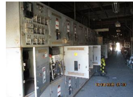
C-633-1 - East Wing Interlor Switchgear Room
