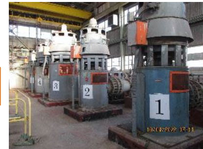
C-633-1 - Center Structure Pumps
