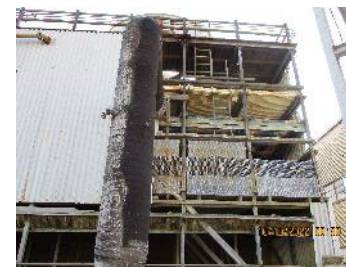
C-633-2B—Interior and Exterior Structural Damage
