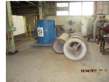
C-633-1 - Center Structure No. 9 RCW Pump
