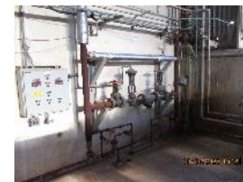
C-633-1 - Center Structure Steam Supply Station
