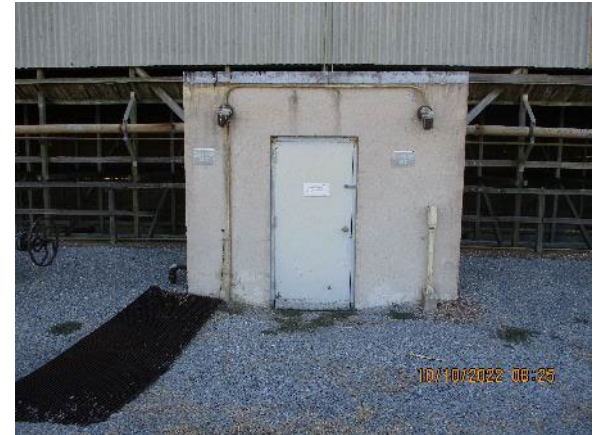
C-633-2B Sprinkler System - External View
