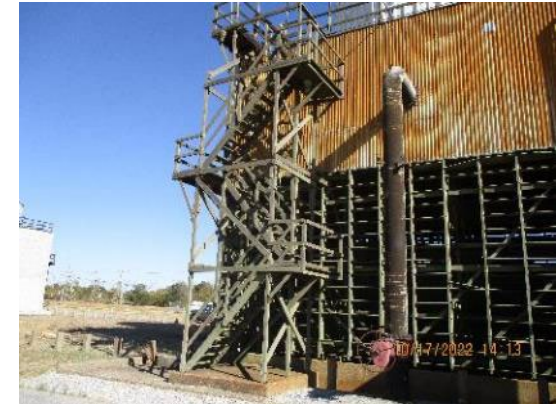
C-633-5 – West Side and No. 9 Riser
