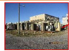
External Electrical Transformers
