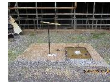
D-Loop Return to Blending Tower Crossover Vault
