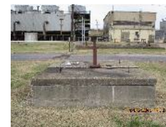
C-Loop Return Bypass to Blending Tower Vault
