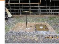
D-Loop Return to Blending Tower Crossover Vault
