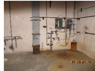
C-633-1 - West Wing Chlorine Fan Exhaust Duct and Metering
