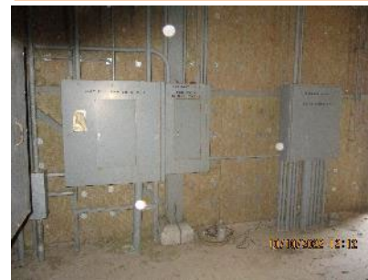
C-633-3 – Electrical Panels
