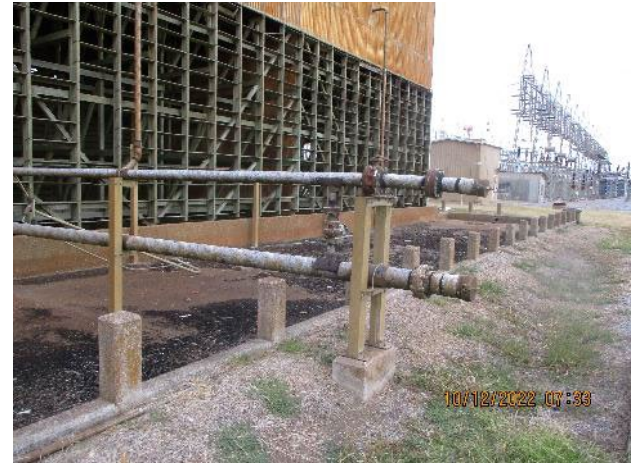
C-633-4 East Side – Flush Line Connection Point
