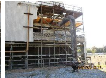
C-633-2A – Southwest Corner Structural Damage
