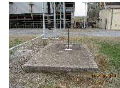
C-Loop Return to Blending Tower Vault
