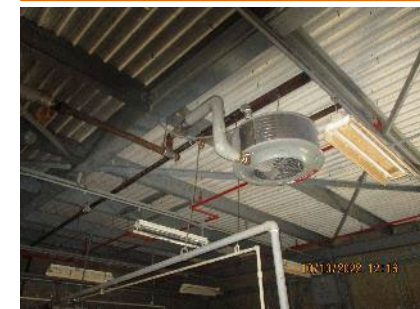
C-633-3 – Steam Heater
