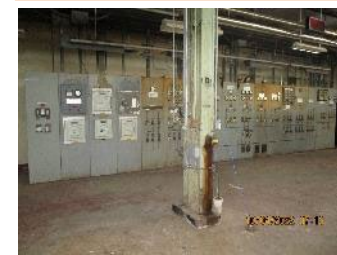
C-633-1 - Center Structure Control Panel
