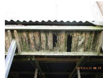
C-633-2B – Interior Structural Damage
