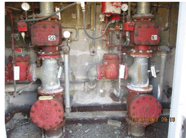
C-633-2A Sprinkler System - Internal View
