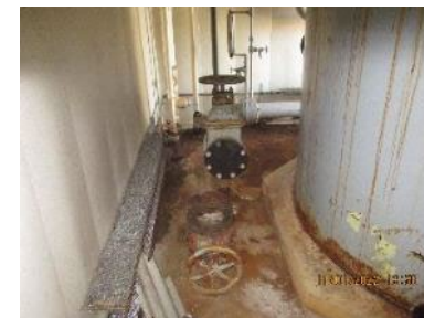
C-633-6 – Sanitary Water Line (Capped)
