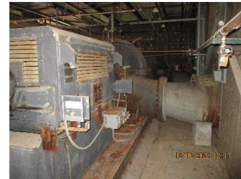
C-633-3 - Pump Suction Line Interior View
