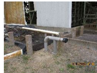
C-633-4 – Fire Protection Connection Point
