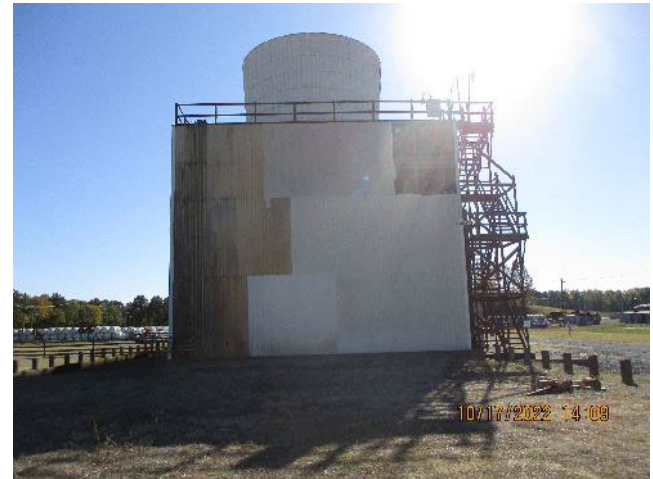
C-633-5 Blending Cooling Tower – North Side
