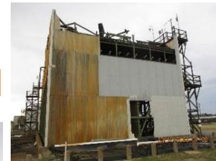
C-633-4 – North Side (Structural Damage)
