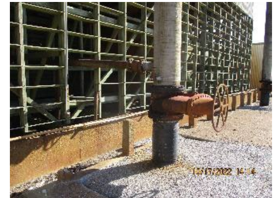
C-633-5 – West Side Riser with Bypass
