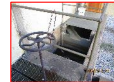
Wet Well Overflow/Blowdown Vault
