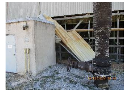
C-633-2A Cooling Tower Loose Fallen Structural Panels
