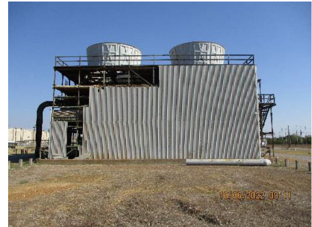
C-633-2A Cooling Tower – South Side
