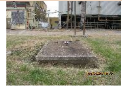
D-Loop Return to Blending Tower Vault
