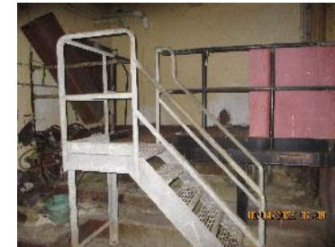
C-633-1 - West Wing Sulfuric Acid Storage and Feed Area
