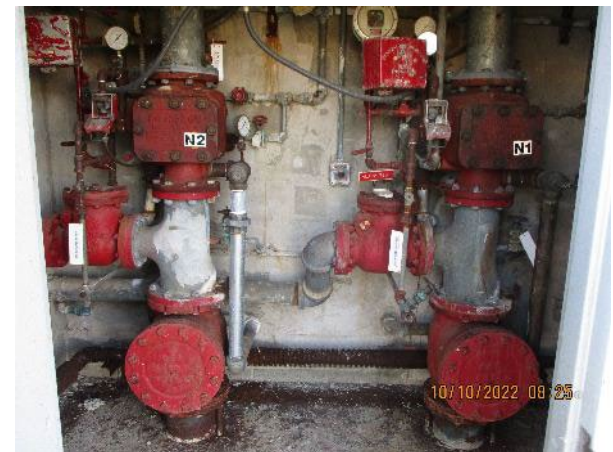
C-633-2B Sprinkler System - Internal View
