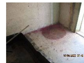
C-633-1 - West Wing Chlorine Room Manhole Cover
