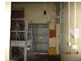
C-633-1 - West Wing Safety Shower
