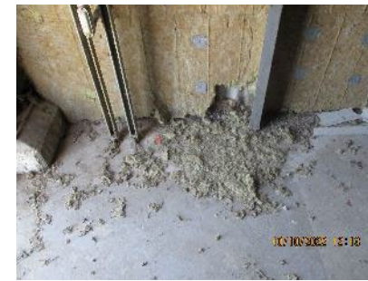
C-633-3 – Damaged Insulation
