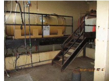
C-633-1 - West Wing Calgon Room (Corrosion Inhibitor Feed Area)
