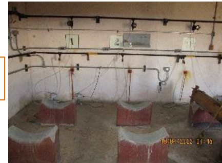
C-633-1 - West Wing Chlorine Feed Header
