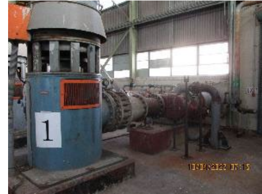
C-633-1 - Center Wing No. 1 RCW Pump and Discharge Lines
