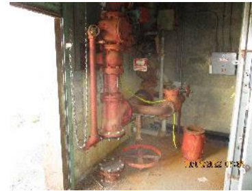
C-633-1 - East Wing Transformer Sprinkler System
