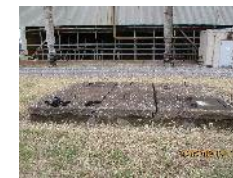
High Pressure Fire Water Valve Vault
