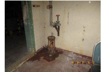
C-633-1 - East Wing Sanitary Water Supply
