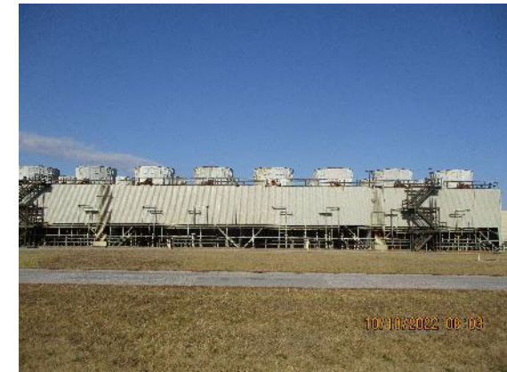
C-633-2B Cooling Tower – East Side
