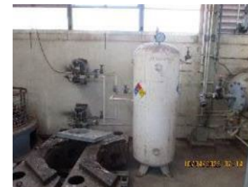
C-633-1 - Center Structure High Pressure Air Tank
