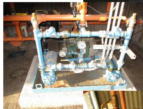
Interior Oil Transfer Pump
