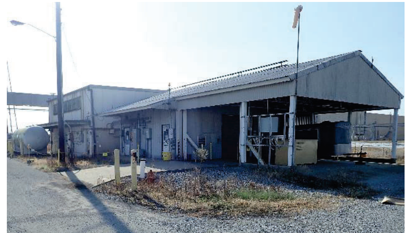
C-410-K Facility Photos: 10/2020
