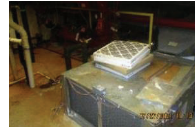
HVAC and floor drain
