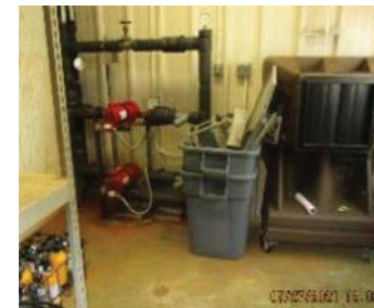
Chilled recirculating water system and floor drain
