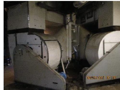
Heat Exchangers and Air Movers in Central Equipment Room
