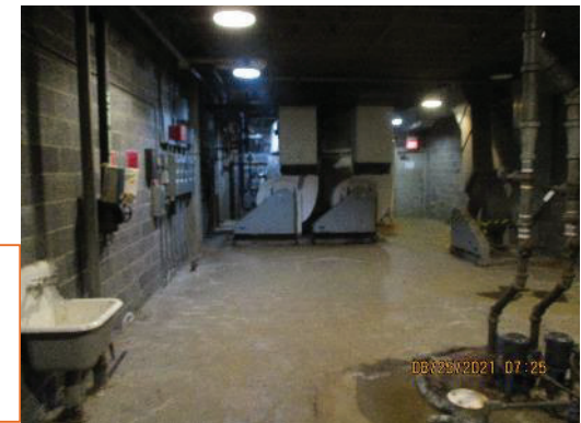
Heat Exchangers, Air Movers, X-Fan in Northeast Equipment Room
