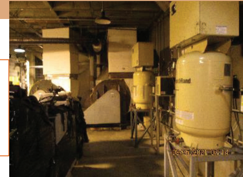
Air Compressor Tanks in Southwest Equipment Room
