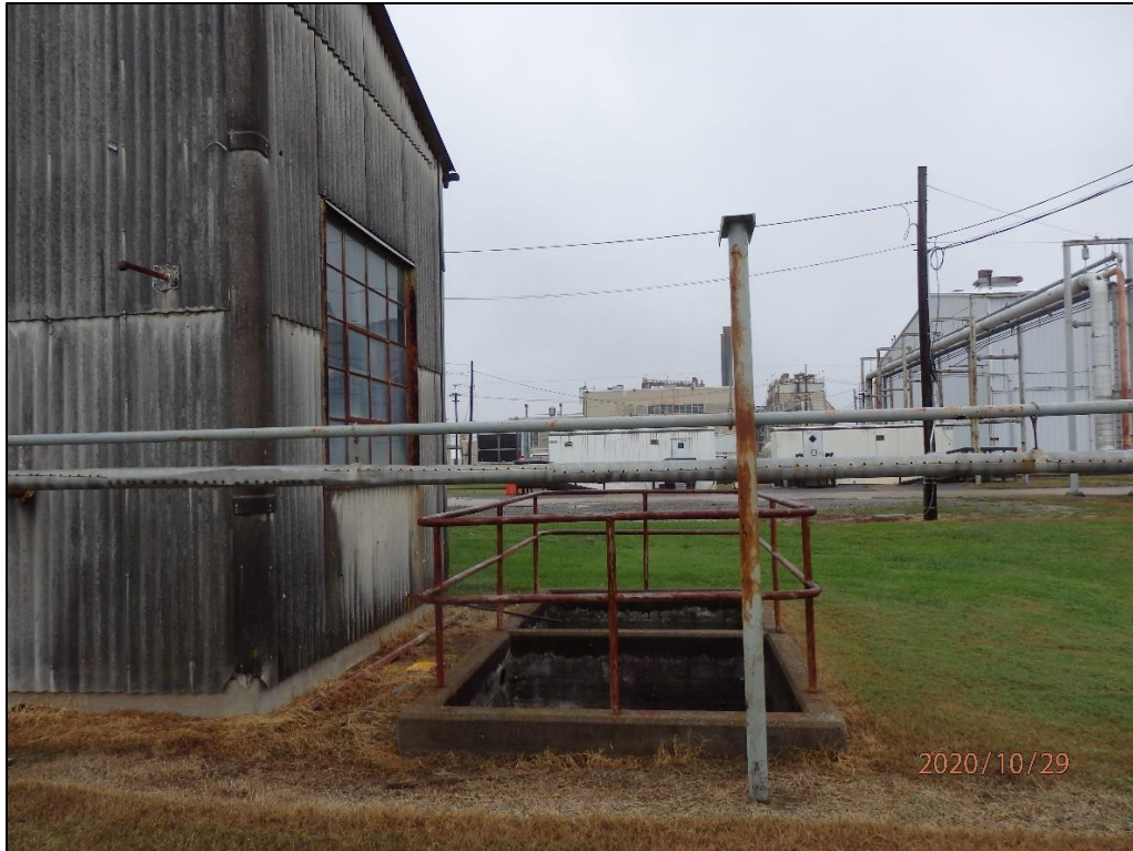
Figure 5. View of East Side of C-729 Showing the SWMU 170 Drain Pits (Looking North)
