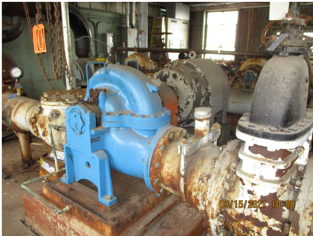
Figure 7. Interior View of C-611-P Looking Northeast Showing the No. 2 Booster Pump and Piping
