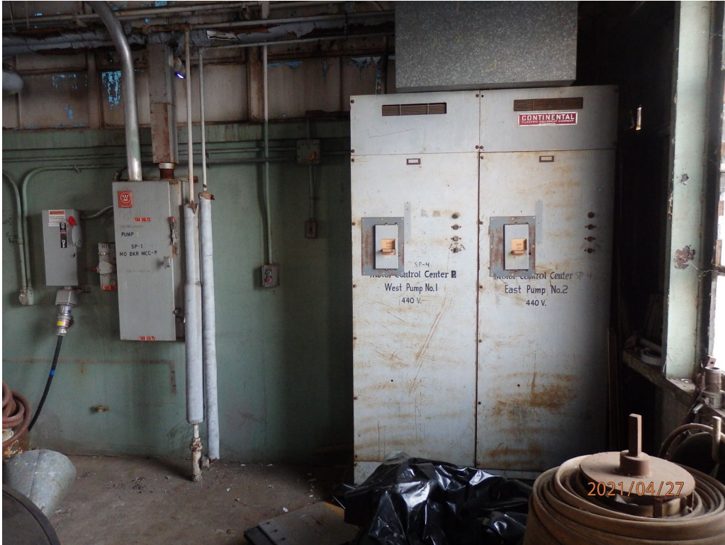
Figure 8. Electrical Switchgear for the Booster Pump Motors
