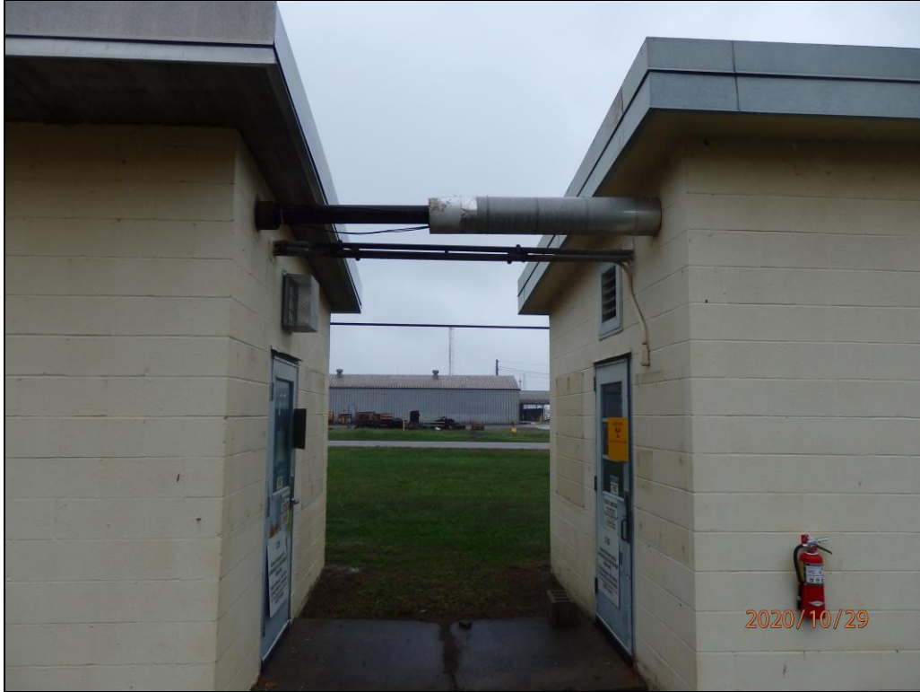
Figure 5. Aboveground Piping Connecting the C-350 Structures (Looking North)
