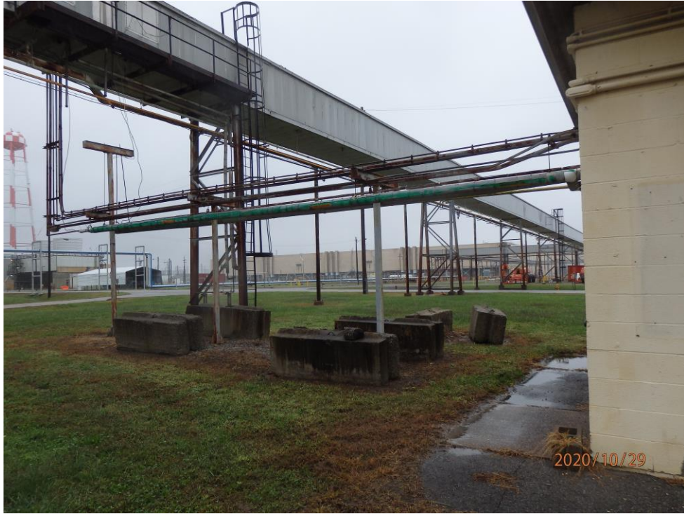
Figure 8. Distribution Piping (Looking East)
