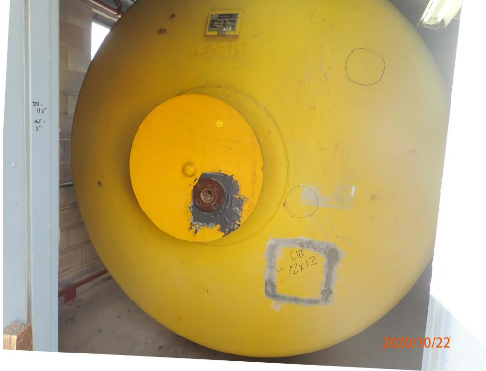
Figure 11. West Mixed Gas Storage Tank
