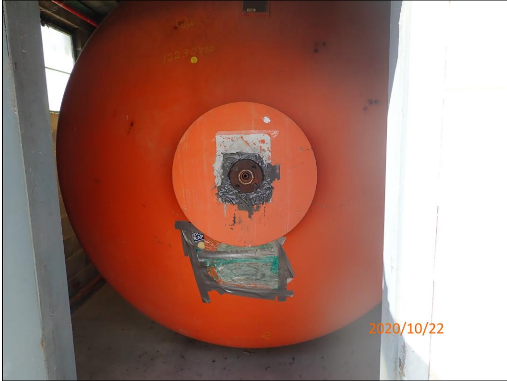
Figure 10. East Mixed Gas Storage Tank
